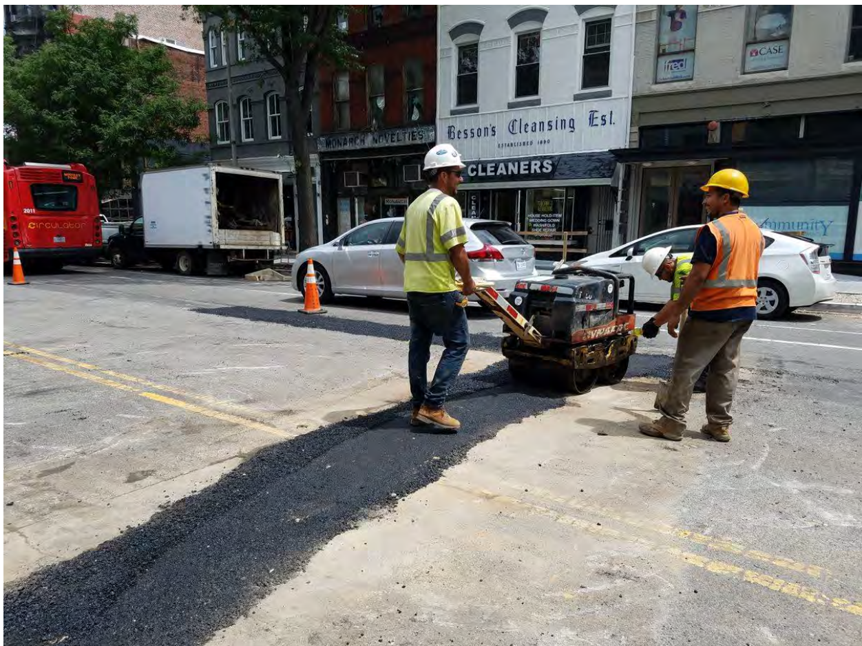
Placing Temporary Asphalt over the lateral trenches between N Street and Rhode Island Ave on the Westside
