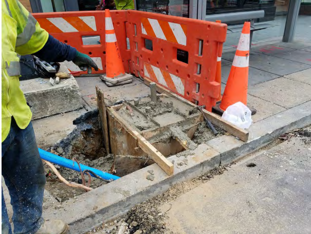
Installation of new Streetlight Foundation between N Street and Rhode Island Ave
