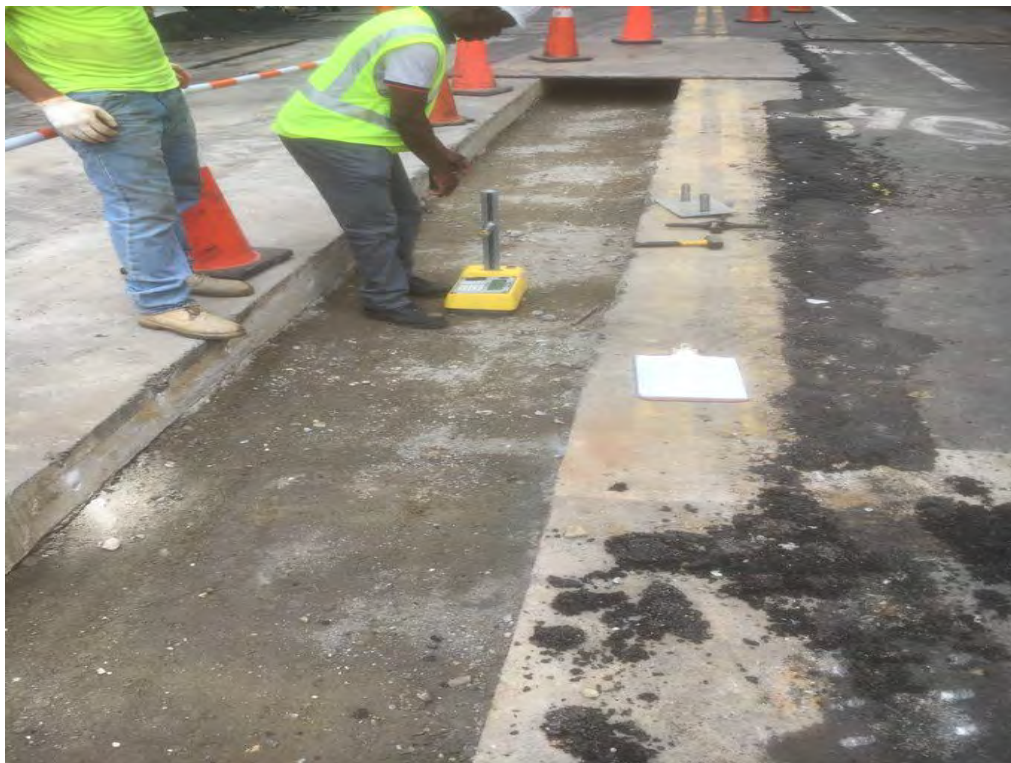
Density Testing of Aggregate Base Material on the Westside of N Street
