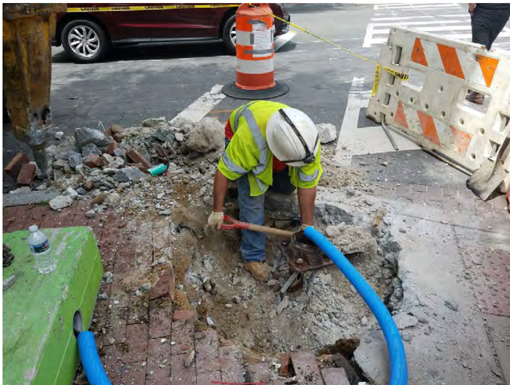
Removal of Existing Traffic Signal / Streetlight Foundation at the SW Corner of Rhode Island Ave
