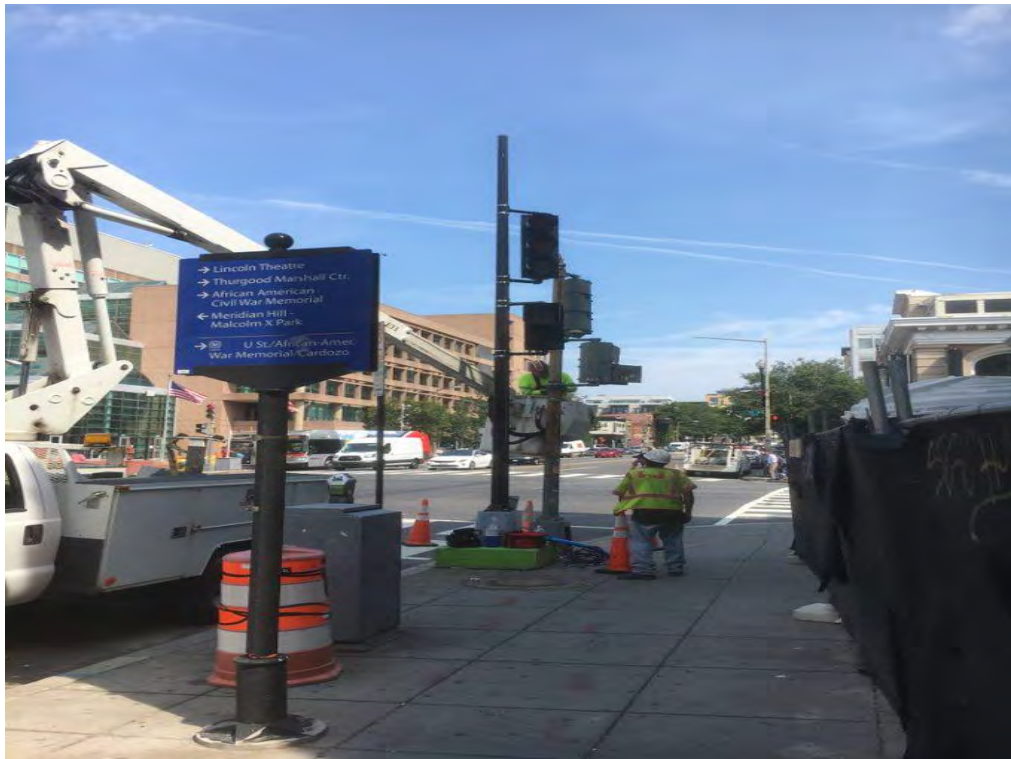
Placement of Temporary Traffic Signal at the NE Corner of 14 th and U Street
