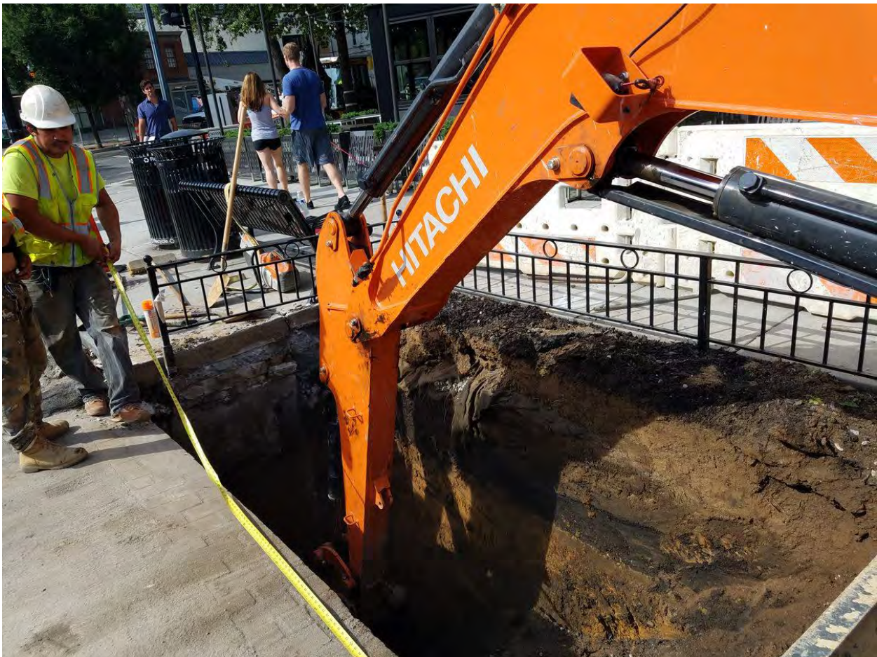
Excavation for Double Catch Basin at Rhode Island Ave on the Westside
