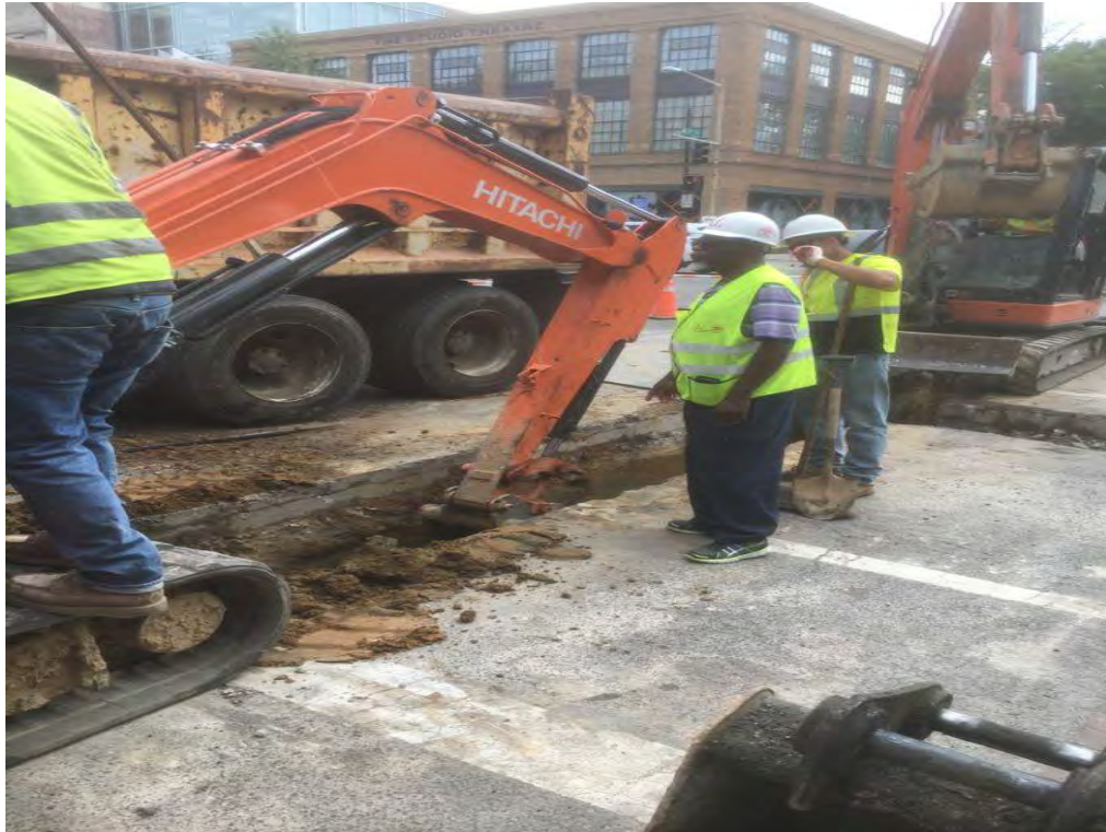
Excavation for 4" and 2" PVC Conduit at the intersection of 14 th and P Street
