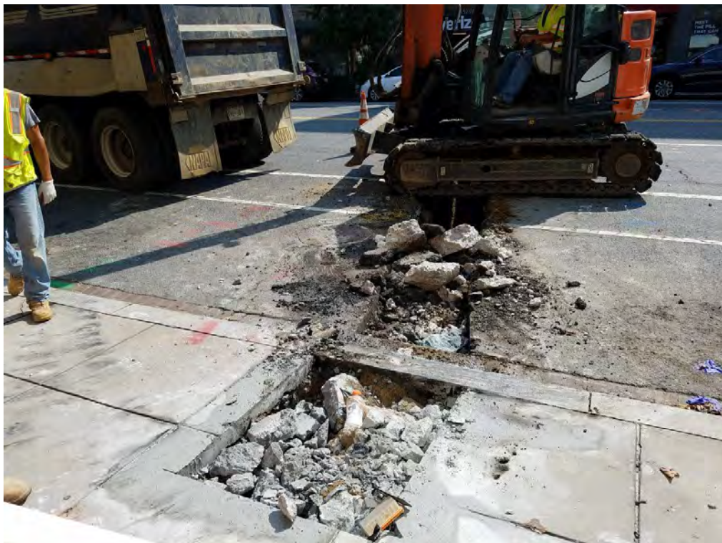
Excavation of Lateral and Street Light Foundation between P Street and Church St.
