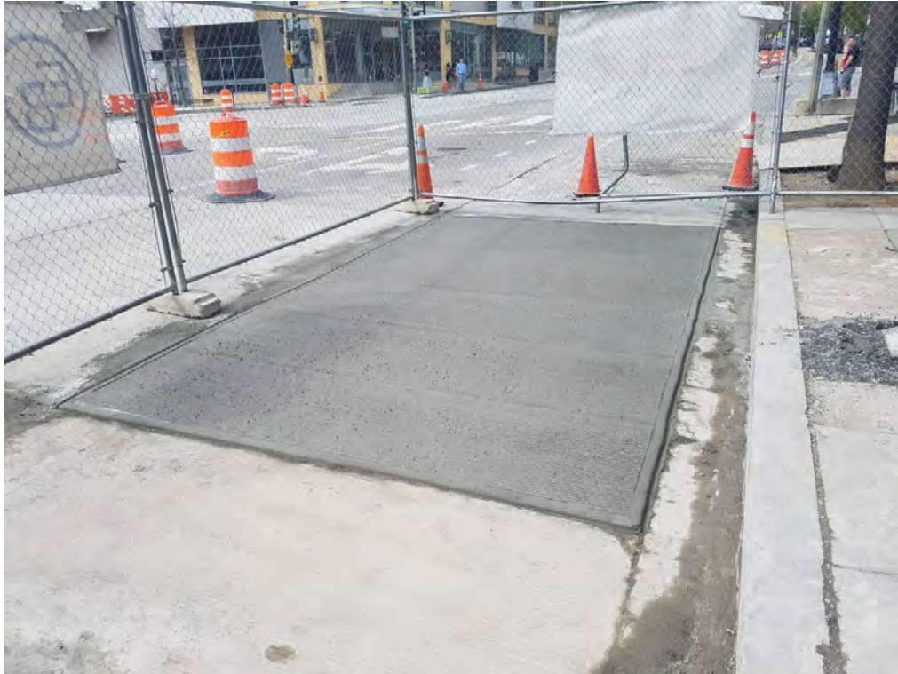
PCC Pavement Repair at the SE Corner of 14 th and W Street
