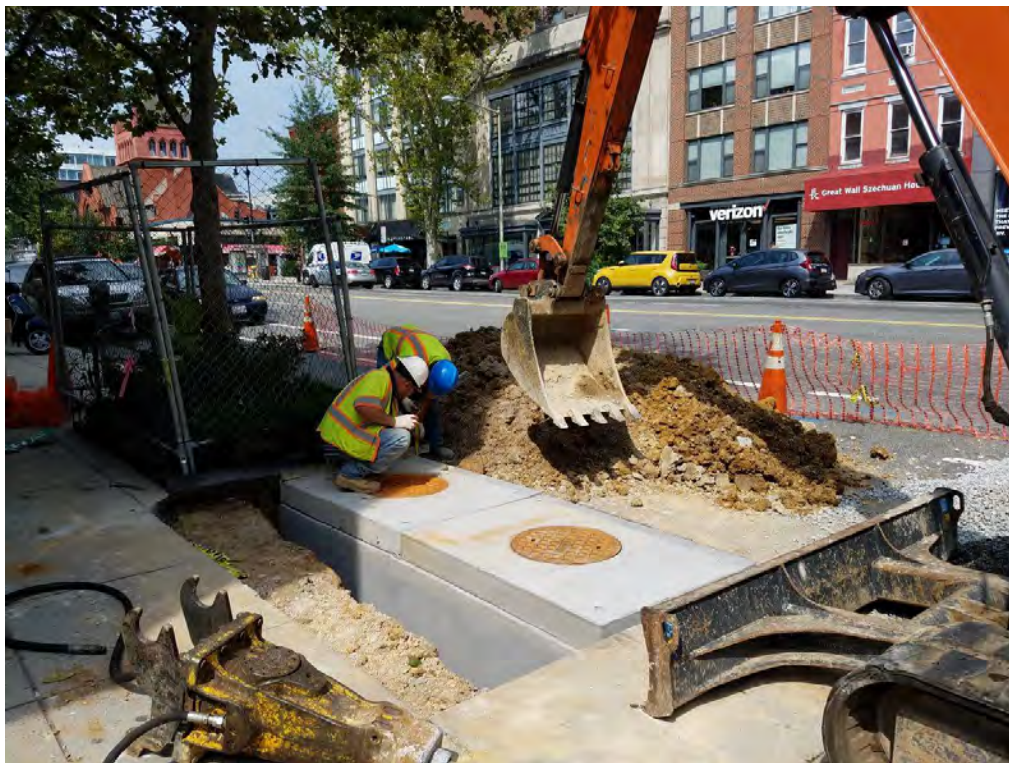
Installation of Double Catch Basin (CB-09) at the NW Corner of Church Street
