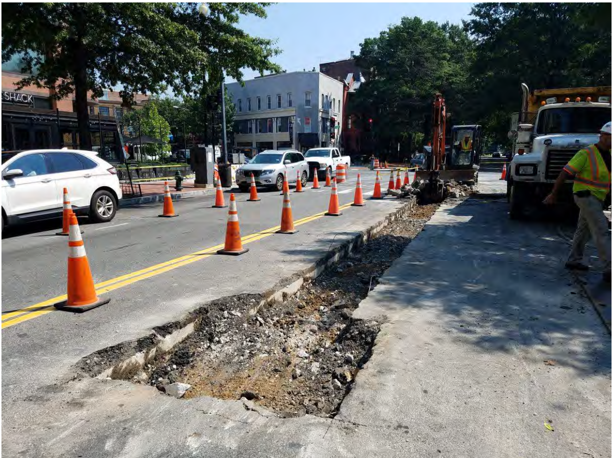
Excavation for Manhole and PVC Conduit on Rhode Island Ave on the Westside
