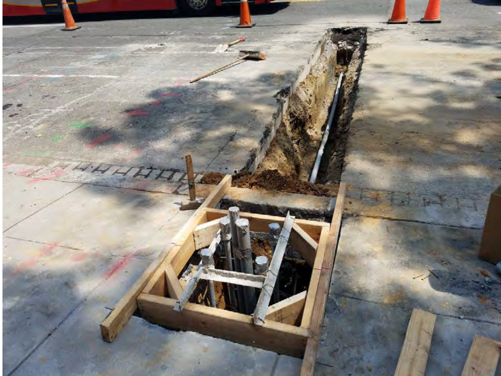
Installation of new Streetlight Foundation between Rhode Island Ave and P Street
