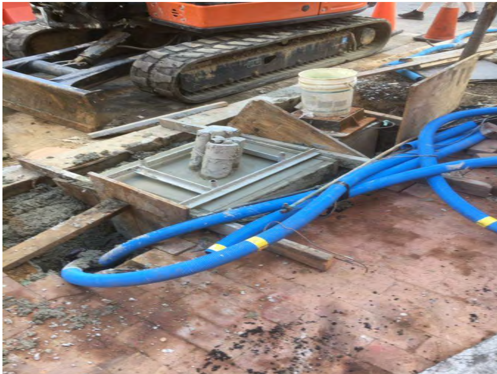
Traffic Controller Foundation at the SW corner of 14 th and N Street
