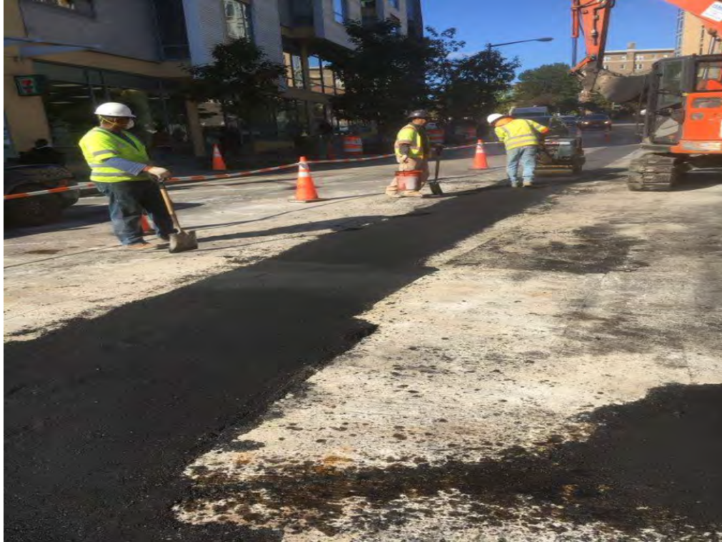
Placement of Temporary Asphalt over Electrical Trench on 14 th at Florida Ave
