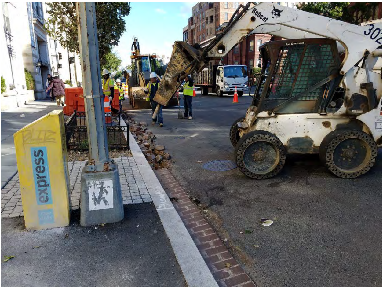
Repairing Brick Gutter that was placed at the wrong Grade between Thomas Circle and N Street Westside
