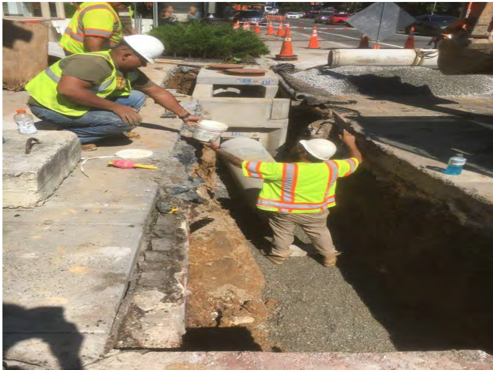
Installation of 15" PCC Connection Pipe for CB-08 at the NW corner of P Street
