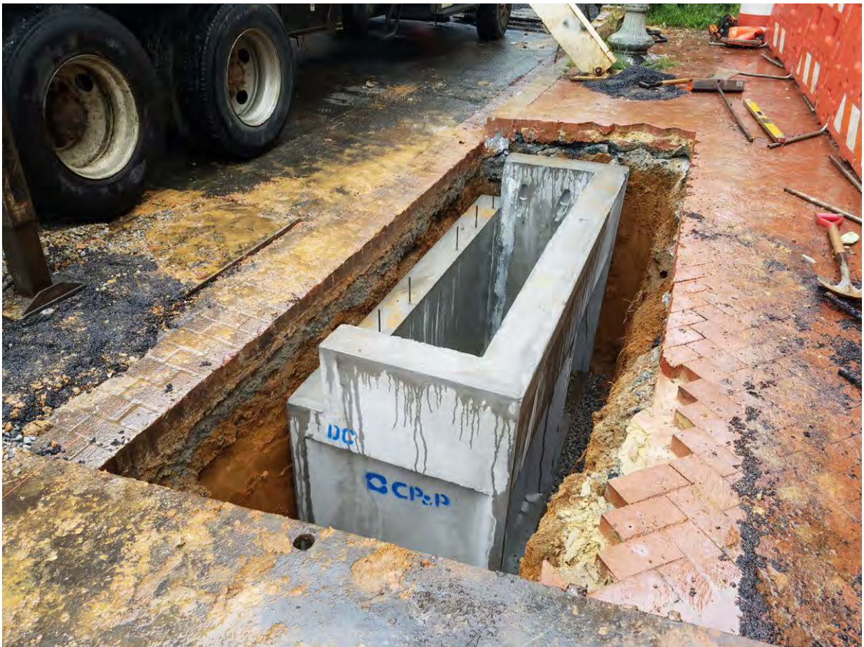
Installing the Double Catch Basin at NW corner of 14 th and Corcoran Street
