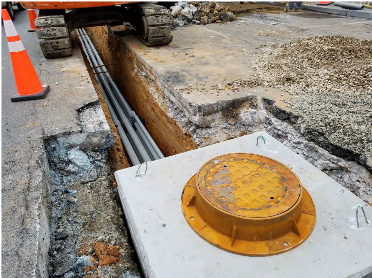
PVC Conduit and Manhole placement between N Street and Rhode Island Ave on the Eastside
