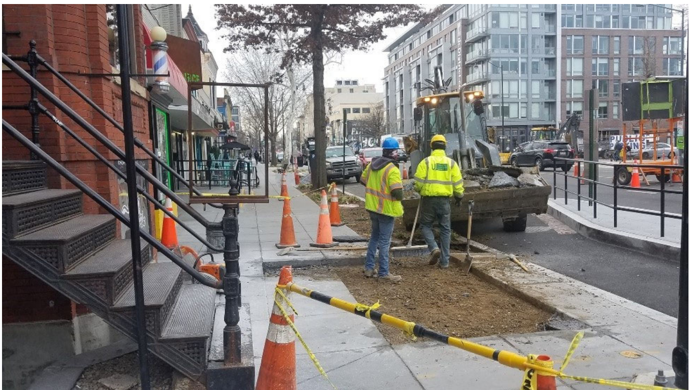
DDOT Contractor worked on repairing the sidewalk at SEC of T Street
