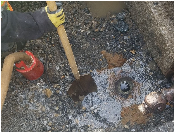
Existing 12" main ruptured by Omni Excavators near T St
