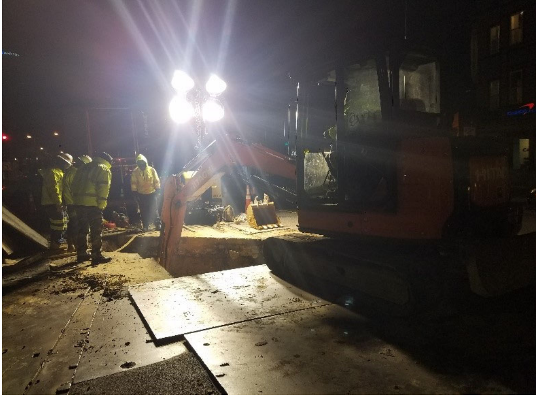
Trench cleared for pipe installation by Omni Excavators at SWC of 14 th & U St
