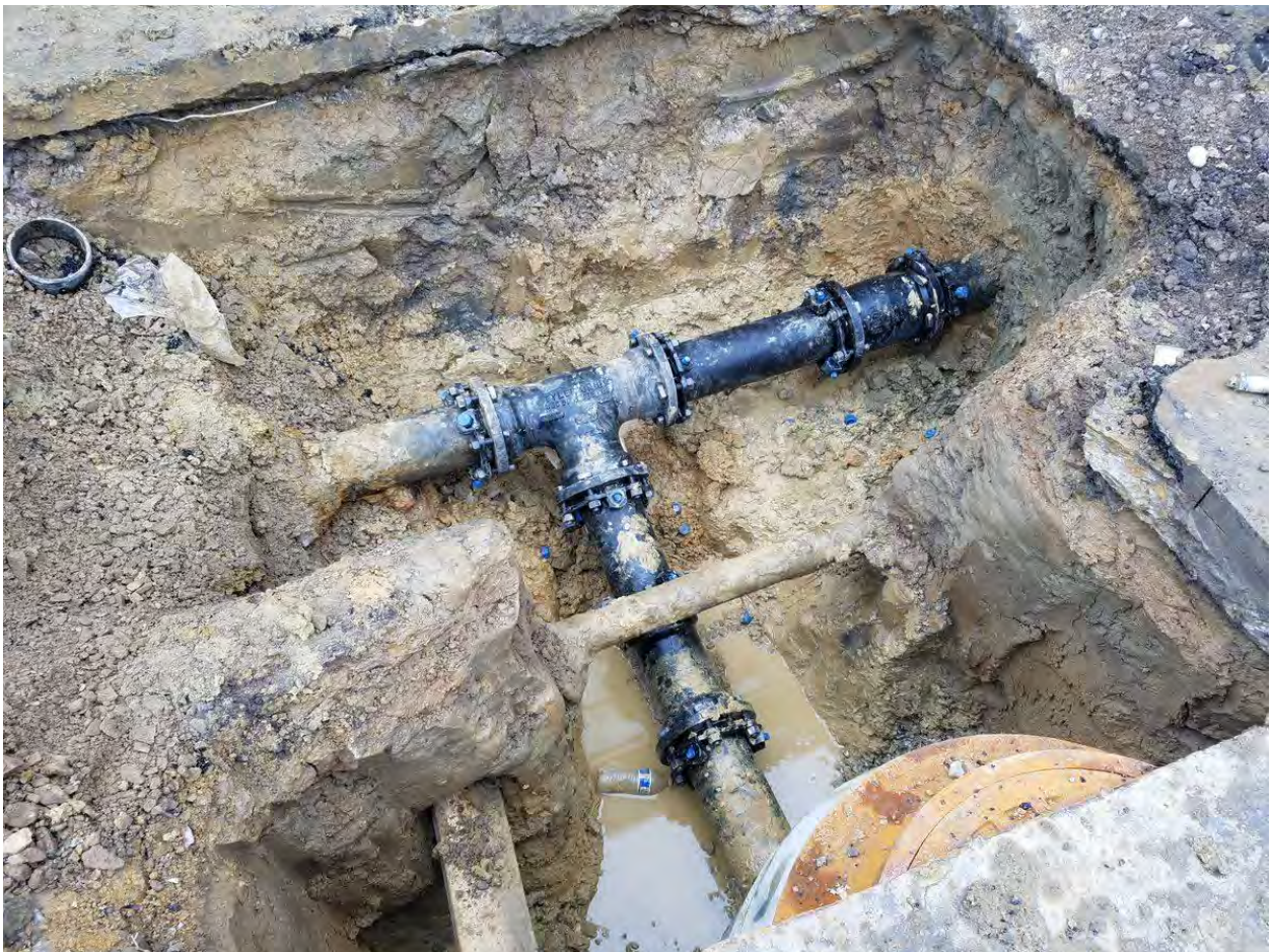
New Water Main and Fire hydrant Connection at 14 th and Swann Street
