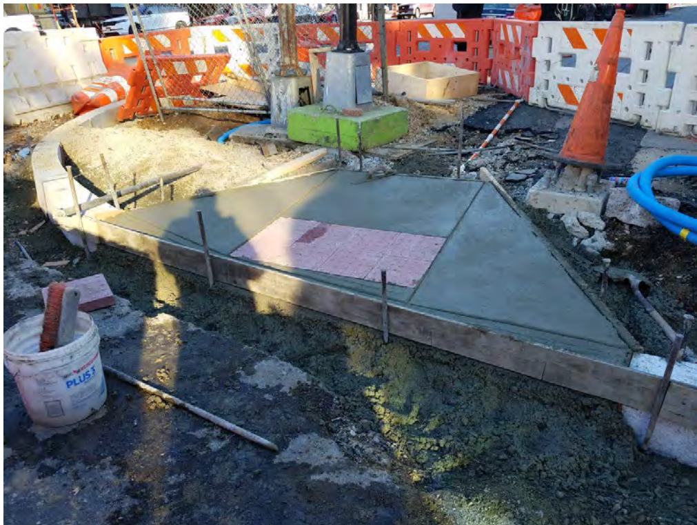
New ADA Ramp at the SE Corner of 14 th and Q Street
