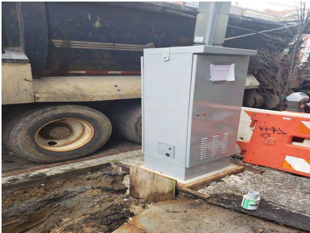
Installation of New Traffic Controller Cabinet
