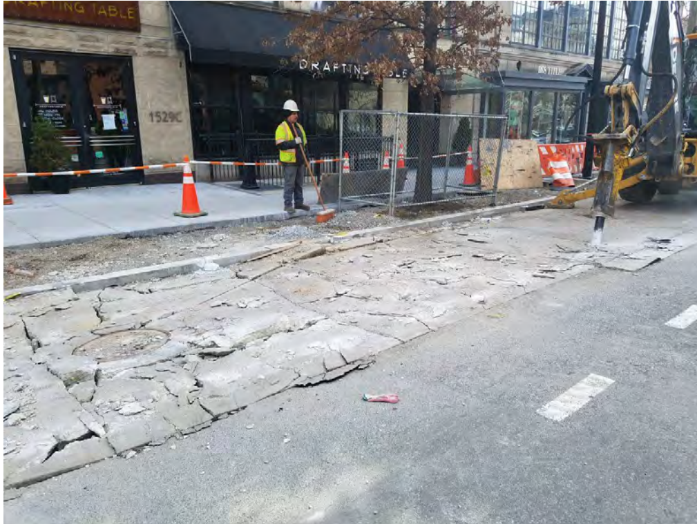
Demo of existing PCC Bus Pad on the Eastside before Q Street
