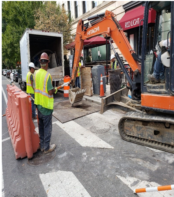
OMNI Inc. crew placed Steel Plate with Cold Patch over the Traffic Signal MH (3'X3'X3') excavation at the Sidewalk at R St. & 14 th St. Intersection at NWC, On Wednesday, 10-2-2019, next to Red Light Restaurant.
