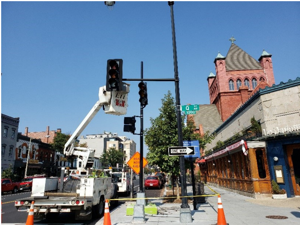
FMCC PePCO crew installed new Signal Lights and removed old Ex. Lights at Q St. & 14 th NW
