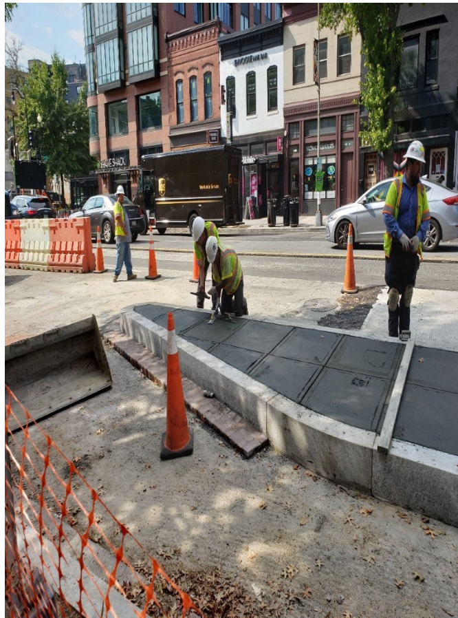
FMCC Concrete Finishers worked on Bus Island after placement of Concrete at Bus Island between R.I. Ave. & P St. NW on 14 th St. NB on Wed. 10-2-2019.
