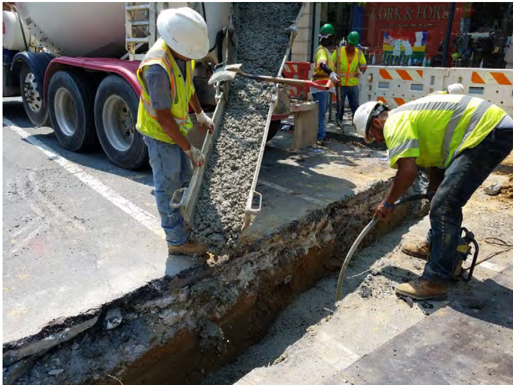
Encasement of 2" PVC Conduit for Lateral between P Street and Church St.
