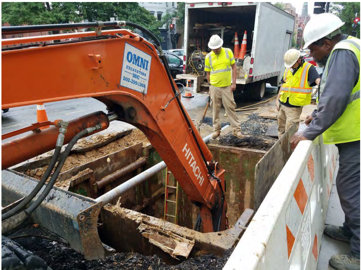
Excavation for Combine Sewer Manhole at Rhode Island Ave on the Westside
