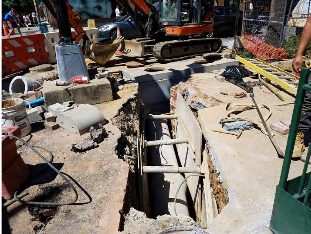
Installation of 15" RCP Connection pipe at SE corner of 14 th and P Street
