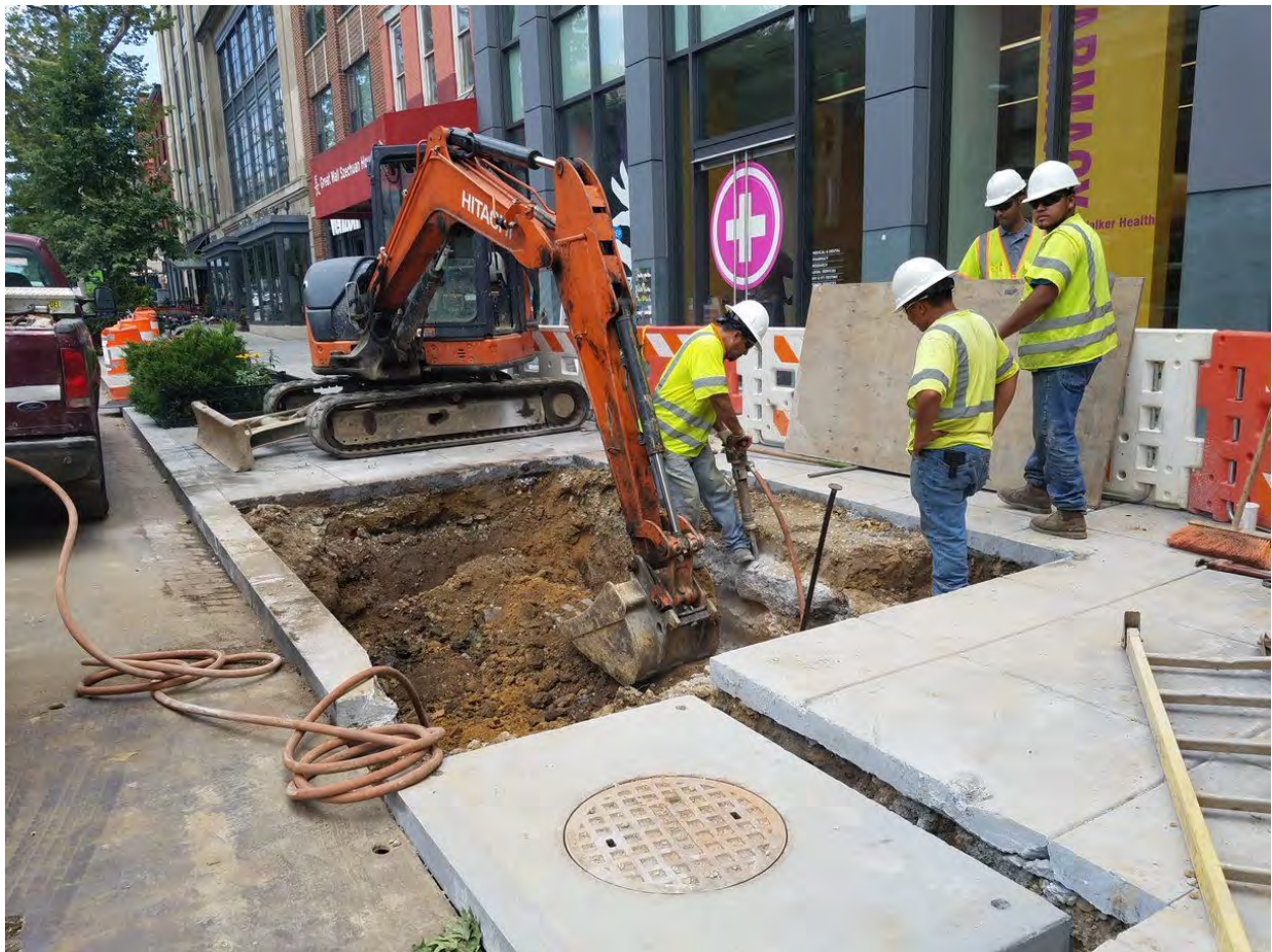
Excavation for Combine Sewer Manhole MH-07 between P Street and Q Street Eastside
