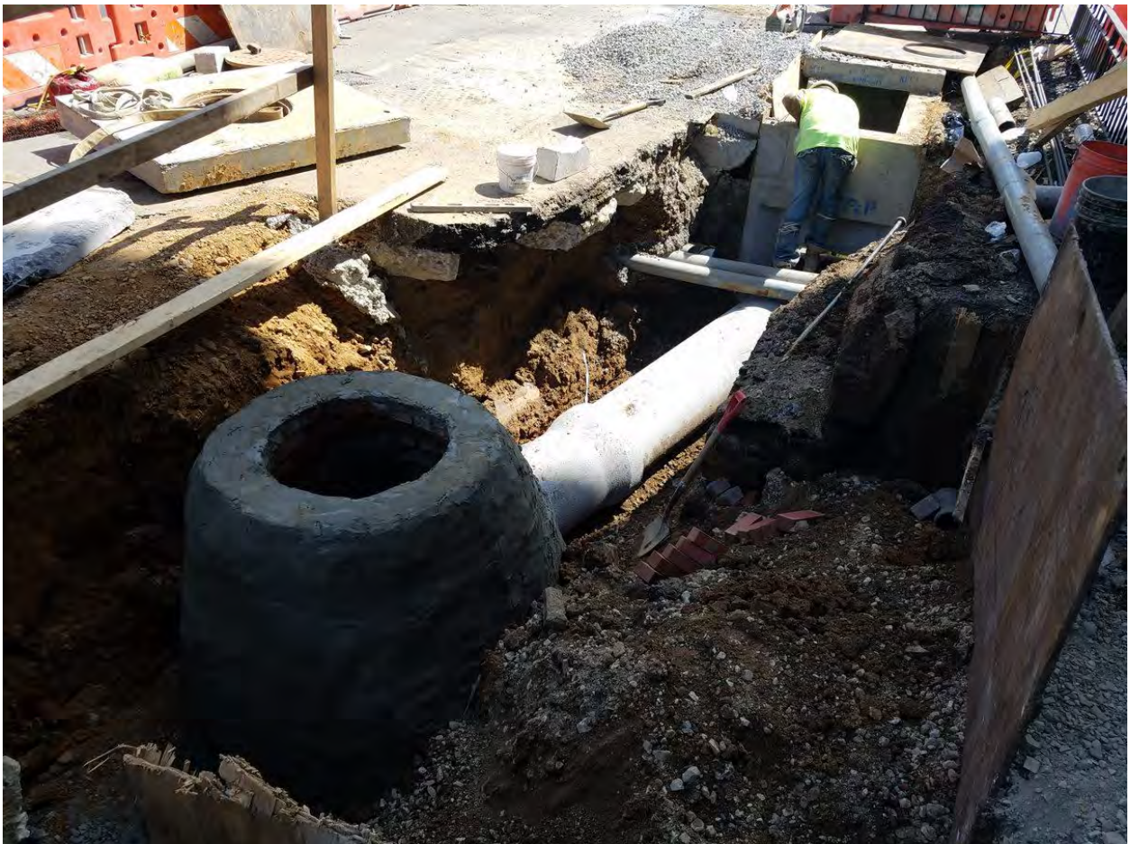
Combine Sewer Manhole and connection pipe to Double Catch Basin at Rhode Island Ave on the Westside
