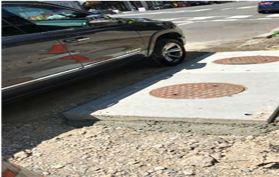
Finished adjusted and poured concrete for the throat and around catch basin top for CB-22.
