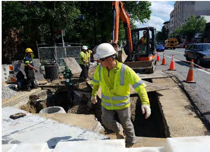
Fire hydrant #H11322 and valve casing installation underway prior to steel plate coverage.
