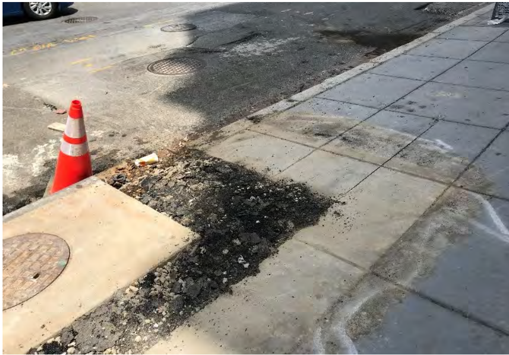
Adjusted catch basin top CB-30 at the NEC of Wallach and 14 th St NW.
