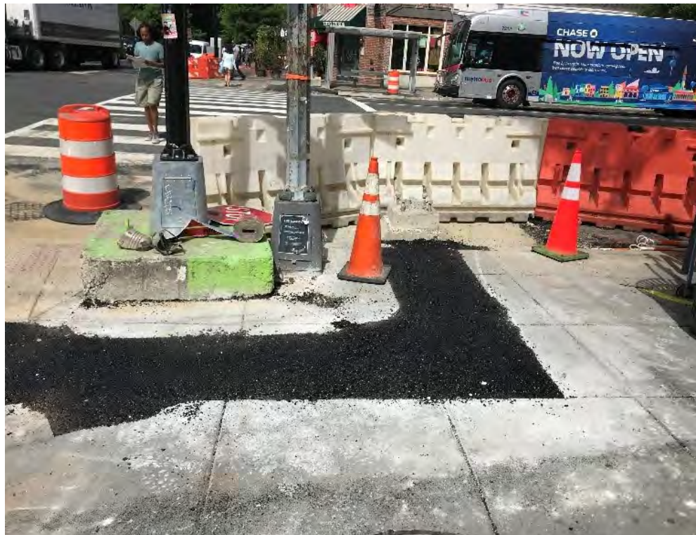
Placed and compacted cold mix asphalt utility trenches at the NEC of 14 th and T St NW.
