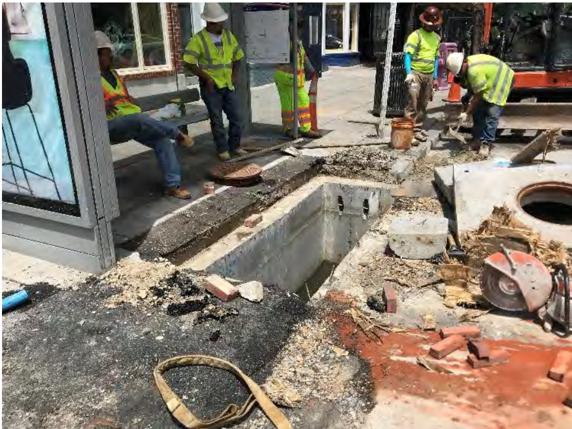
Adjusted catch basin top CB-28 at the NEC of T and 14 th St NW.
