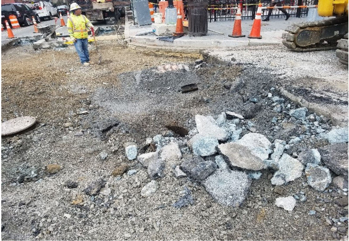
Valve casing abandoned at R ST Intersection
