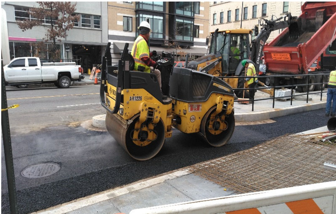
FMCC compacting the surface Mix 12.5MM in the bike lane between Sta 26+53 & Sta 27+79 NB 14 th Street NW
