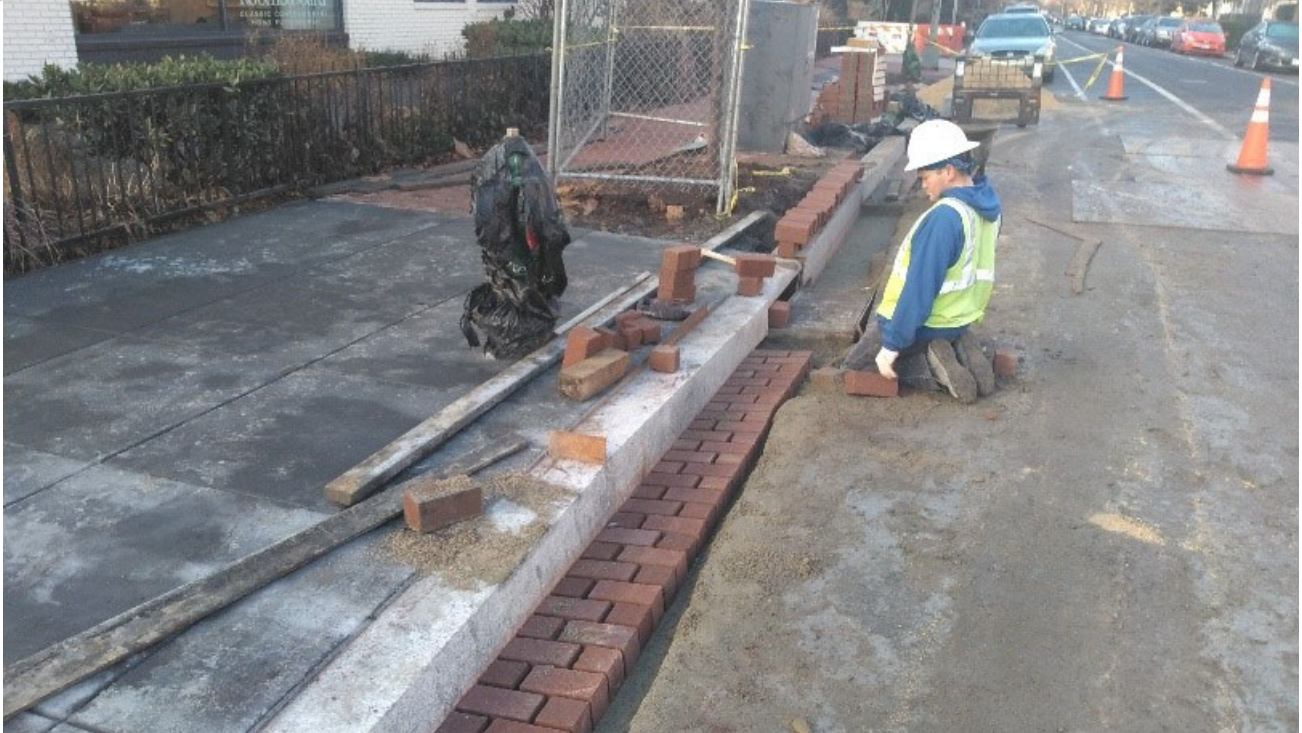
DEN installing the Brick Gutter at the SW corner of T Street & 14 th Street NW
