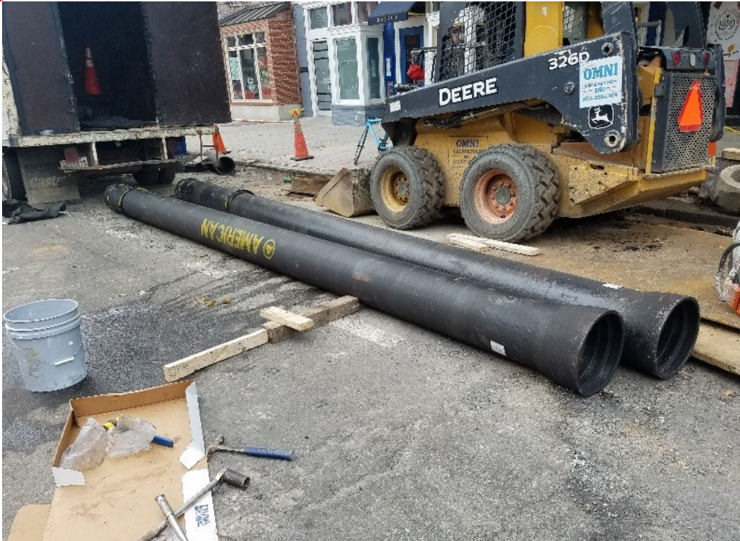
Omni at 14 th St between T St and Wallach St pipe delivered
