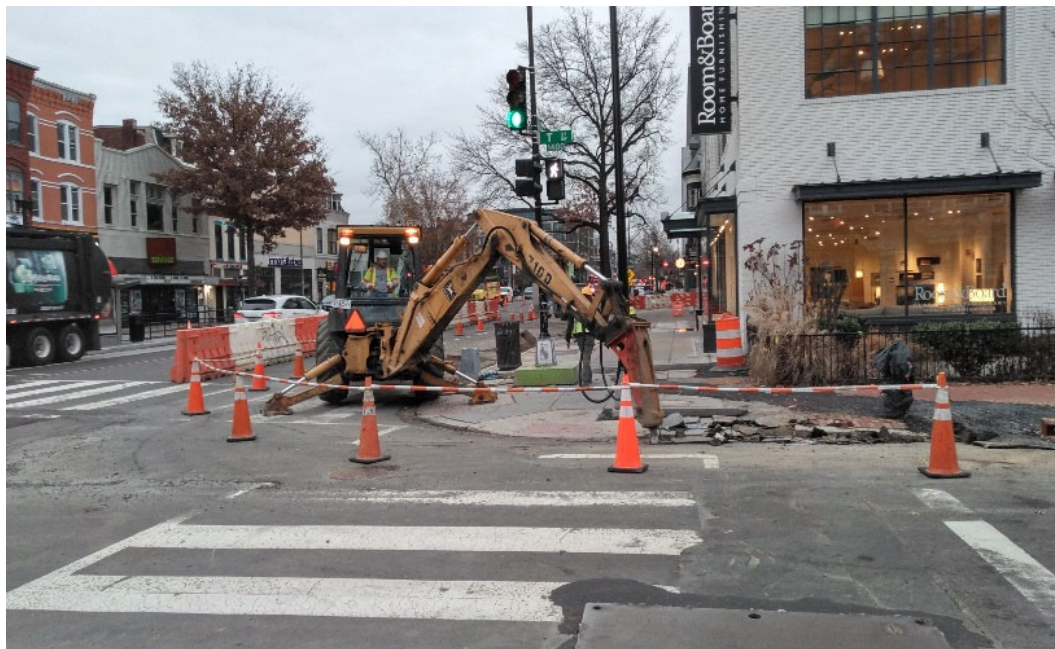
DEN demoing the existing curb, sidewalk and handicap ramp at the SW corner of T Street & 14 th
