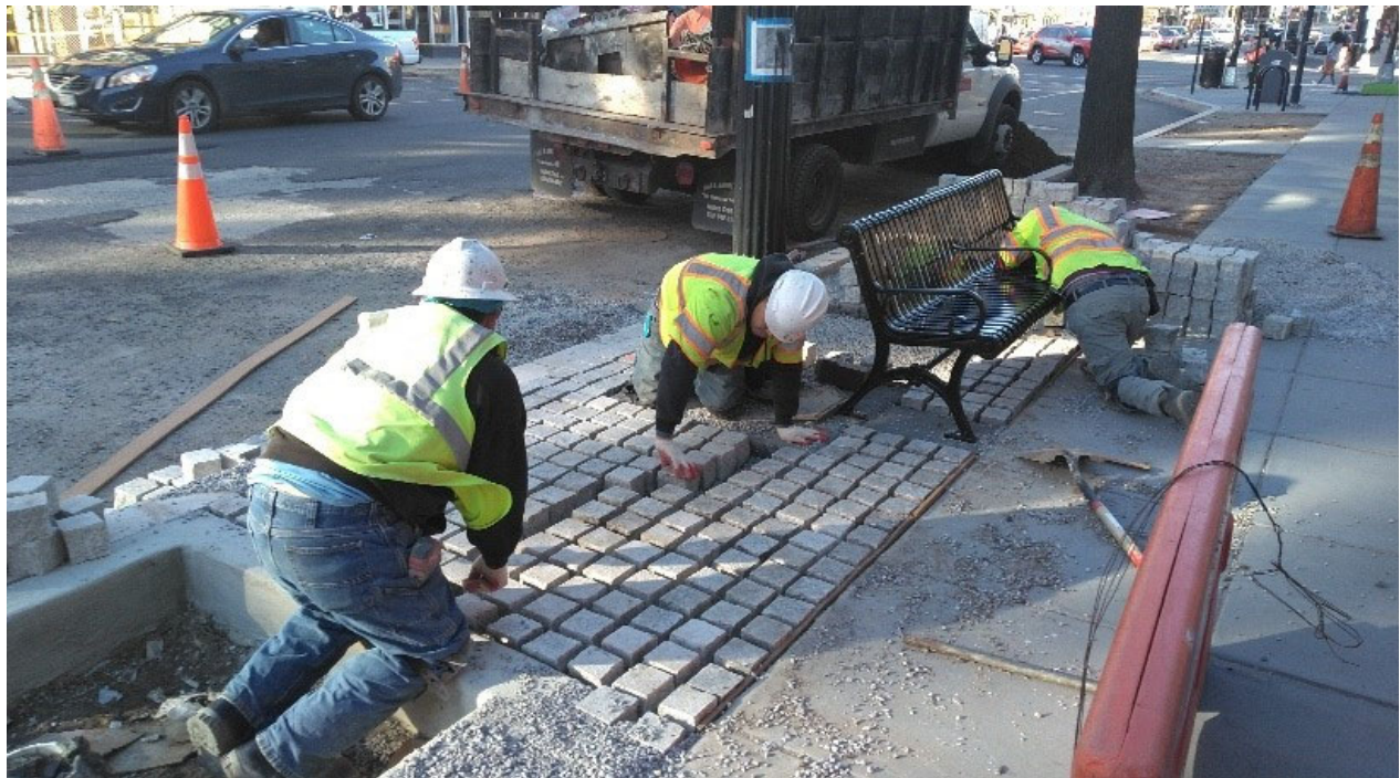
DEN reinstalling the permeable pavers at 1925 14 th Street NW after installing the Geo Grid
