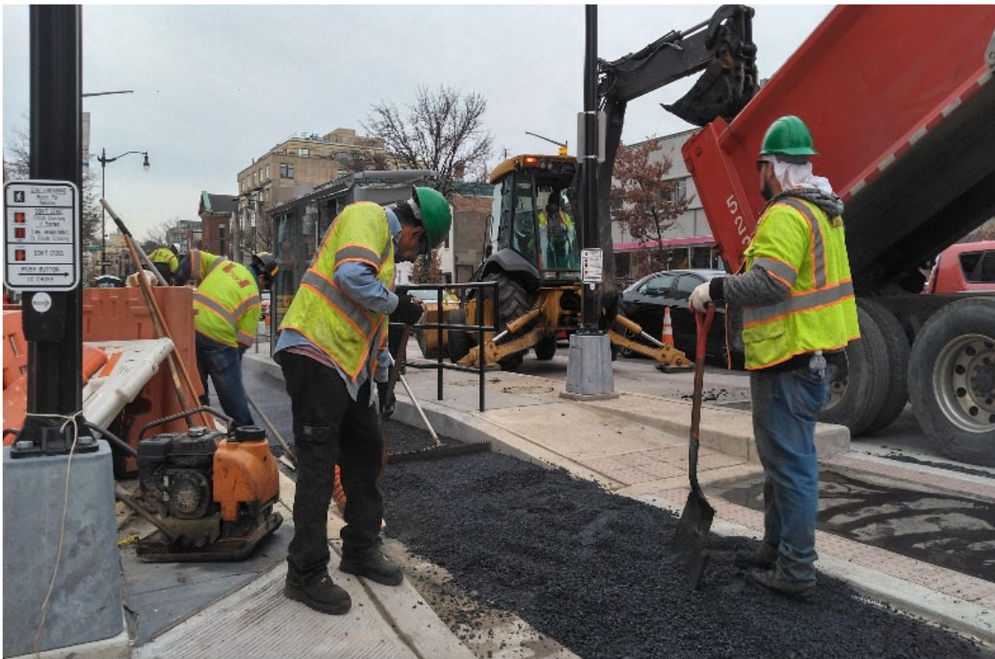
FMCC spreading the 12.5 MM Surface mix by hand in the bike lane between Sta 26+53 & Sta 27+79 NB 14 th Street NW
