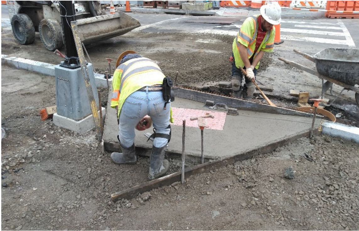
DEN finishing a handicap Ramp at the SW corner of T Street & 14 th Street NW
