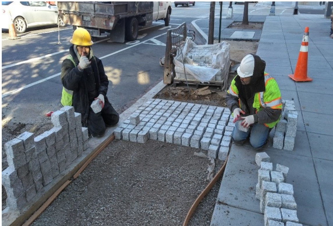
DEN getting ready to place the permeable pavers at 2019 14 th Street NW
