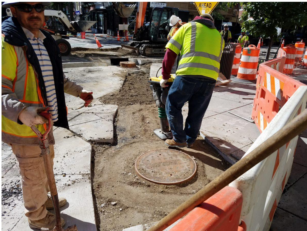
Compaction of material around manhole on Westside of Florida Ave and 14 th Street
