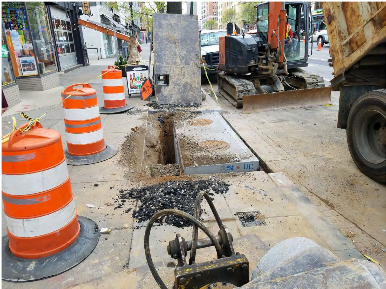
Installation of new Double Catch Basin at the SEC of 14 th and Rhode Island Ave
