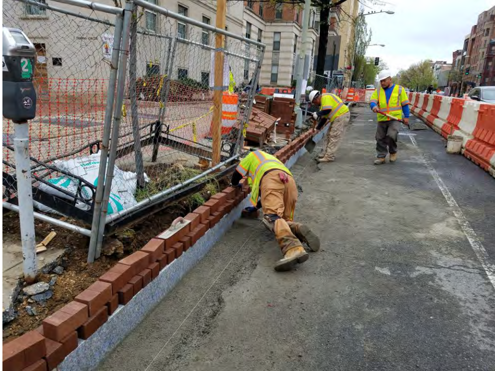
Placing New Brick Gutter on the Westside between Thomas Circle and N Street
