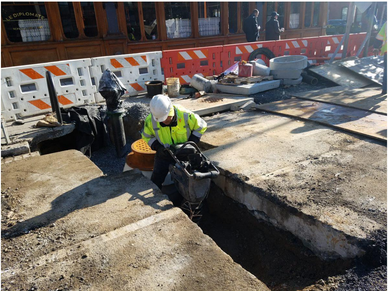
Compacting Backfill for the new Fire Hydrant installed at the NE Corner of 14 th and Q Street
