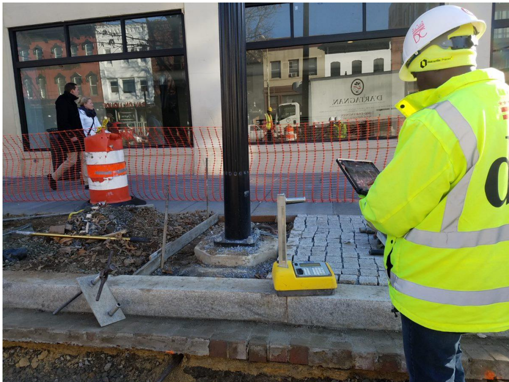
QA/QC onsite to perform Compaction Testing of Aggregate Base prior to PCC Base placement
