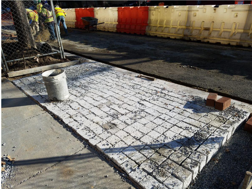
Placement of Cobble Stone Pavers at the NE Corner of 14 th and P Street
