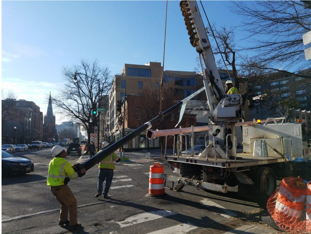
FMCC Electrical installing new Pendant Poles at the SW corner of Rhode Island Ave
