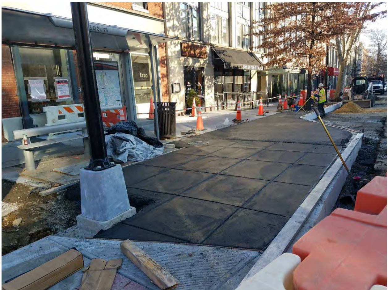
New PCC Sidewalk at the SE corner of 14 th and Q Street
