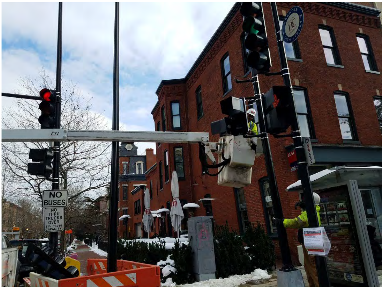
Installation of Pedestrian Signal Head at the NE Corner of 14 th and Q Street
