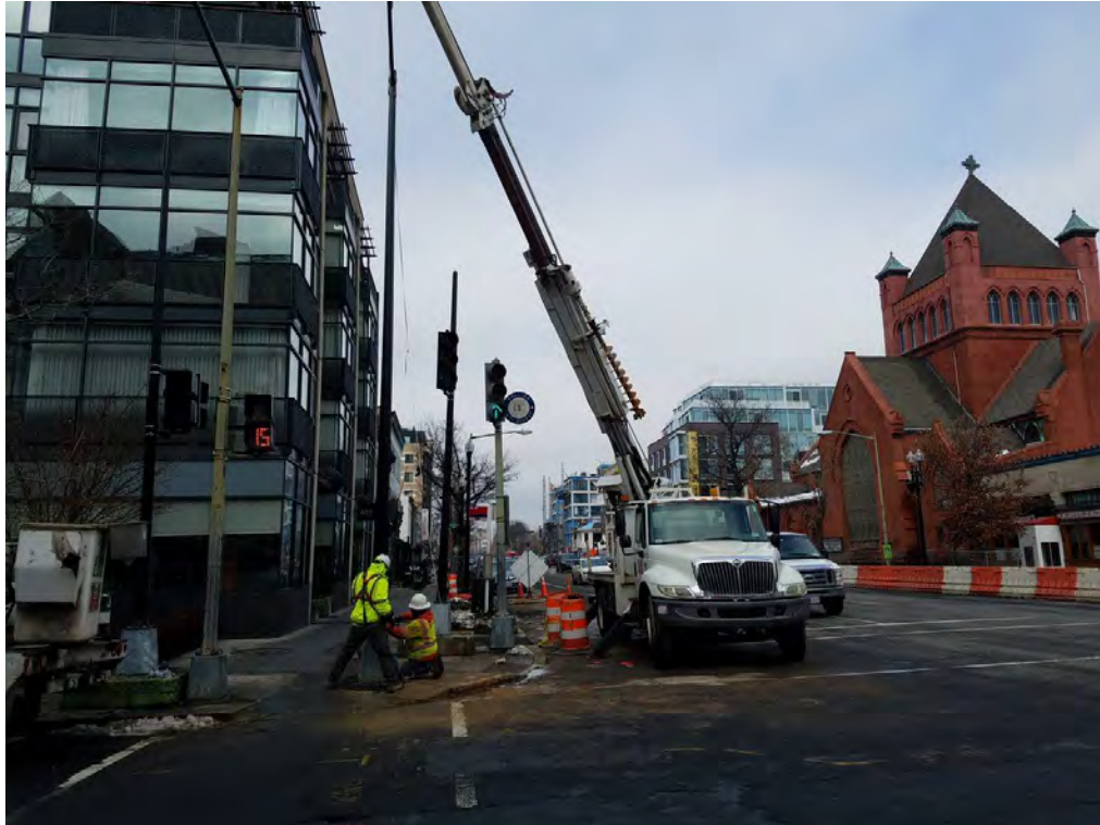
Installation Traffic Signal Pole at the NW Corner of 14 th and Q Street
