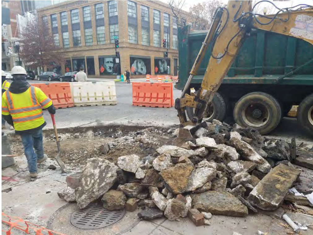
Demo for installation of Bump Out at the SW Corner of 14 th and P Street
