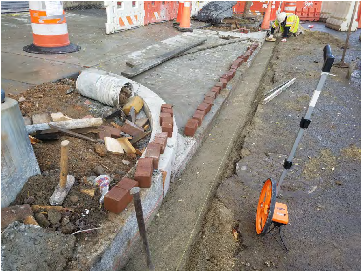
Placement of Brick Gutter between N Street and Rhode Island on the Westside
