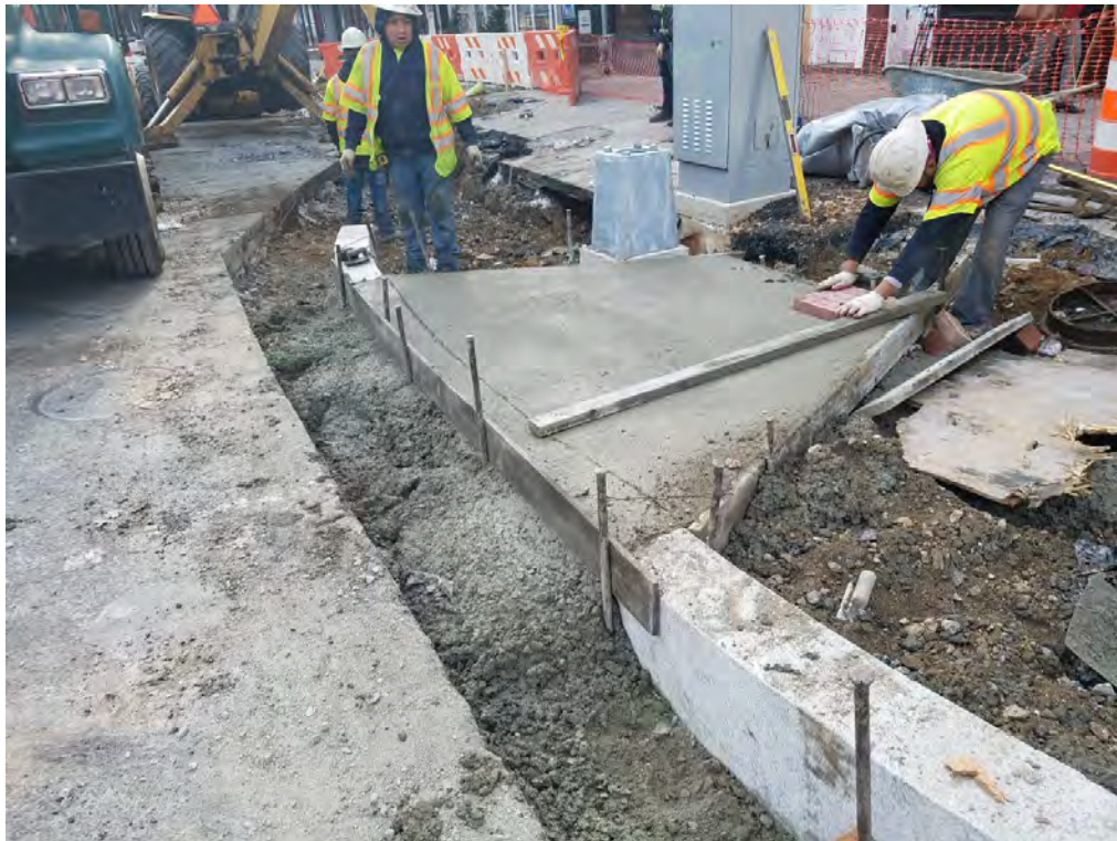
Installation of ADA Ramp at the SW corner of 14 th and P Street
