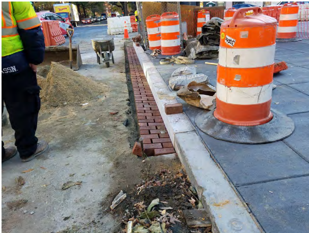
Installation of Brick Gutter SW corner of 14 th and Rhode Island Ave westside
