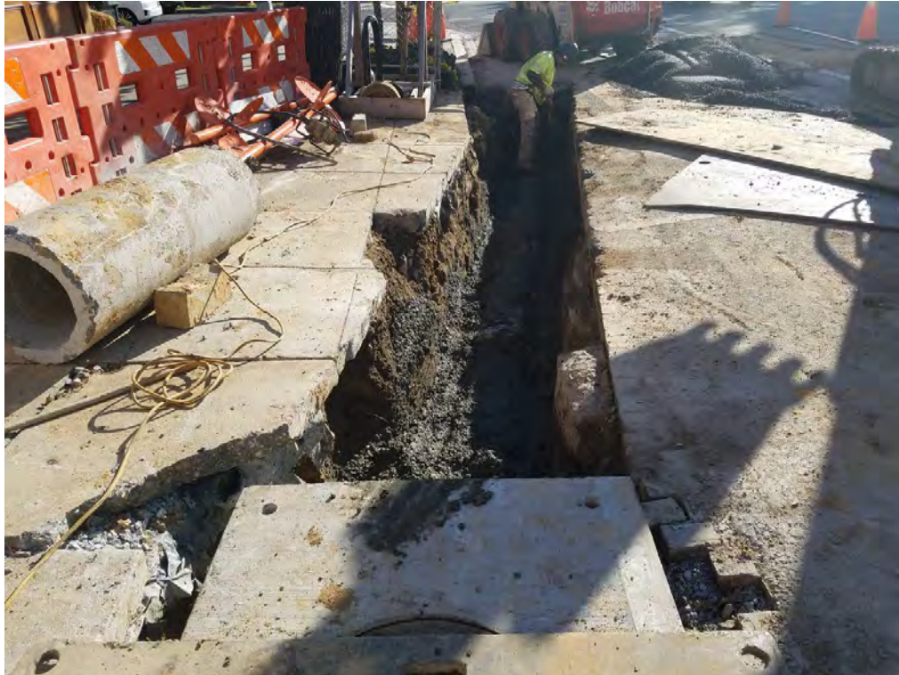
Installation of Combined Sewer connection pipe at the near 14 th and Q Street
