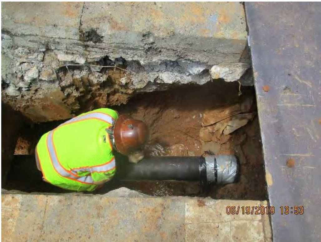
Omni continued the Installation of 8-Inch D.I.P at 14 th & R Street NW
