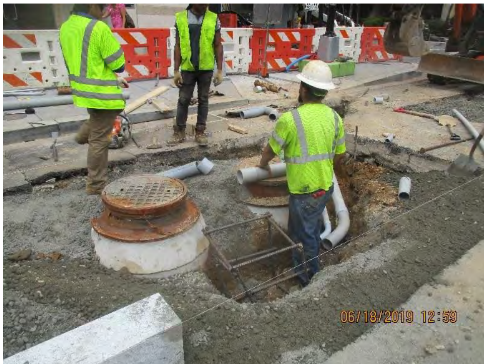
Omni installing the Street Light Pole Foundation TS06 within the area of the proposed Bus Island at 14 th & N Street NW
