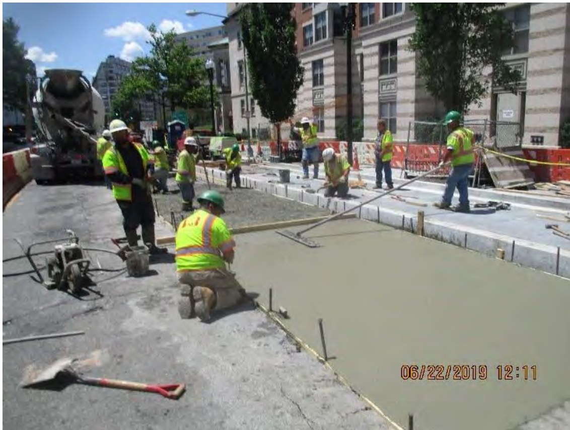
FMCC finishing up the concrete work for the installation of the Bus Pad at the southwest corner of 14 th & N Street NW
