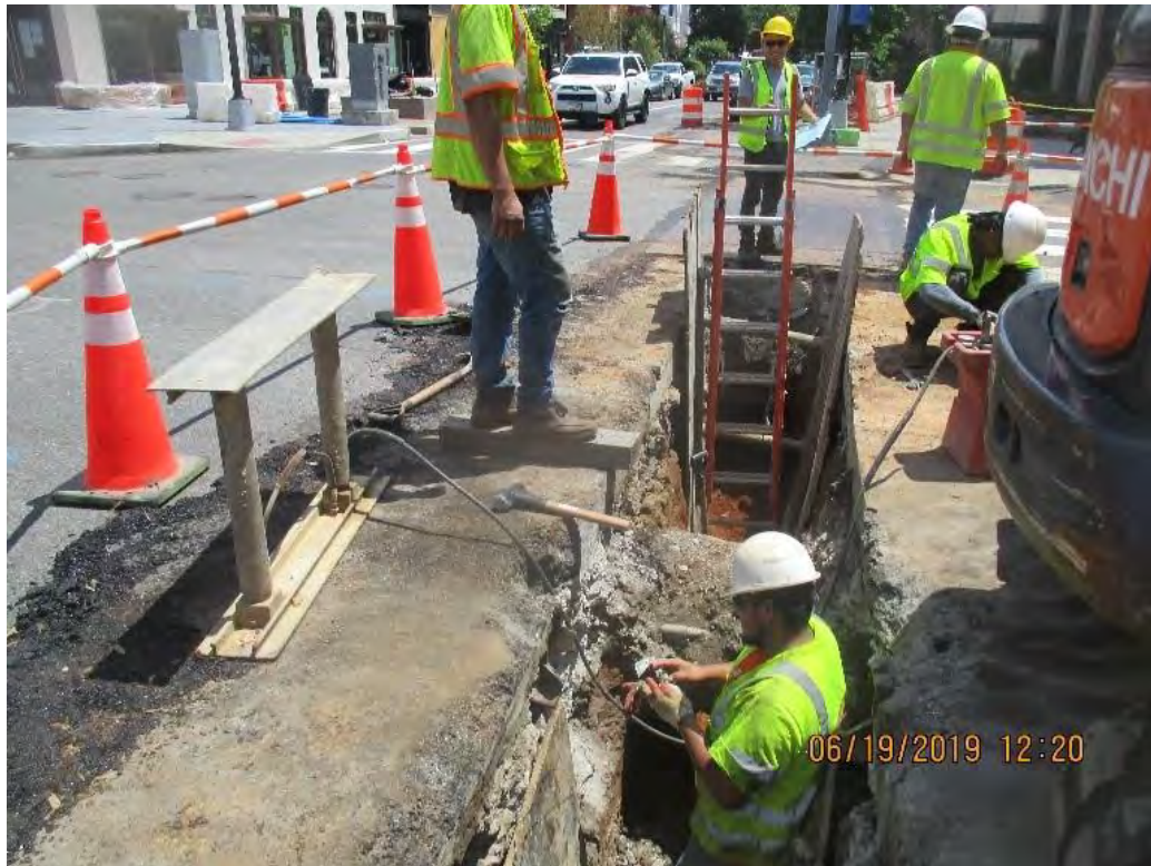
Omni continued the Installation of 8-Inch D.I.P at 14 th & R Street NW
