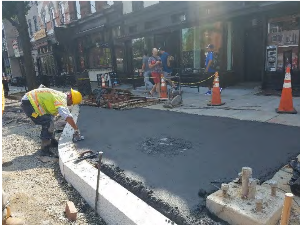
PCC sidewalk at SWC of 14 th 7 Corcoran St finishing underway by D.E.N.
