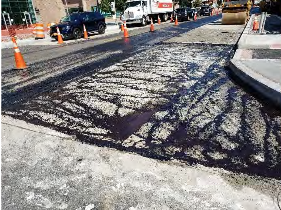
FMCC Asphalt placed Tack next to Bus Island at 2001 block of 14 th St. NW in NB Direction.
