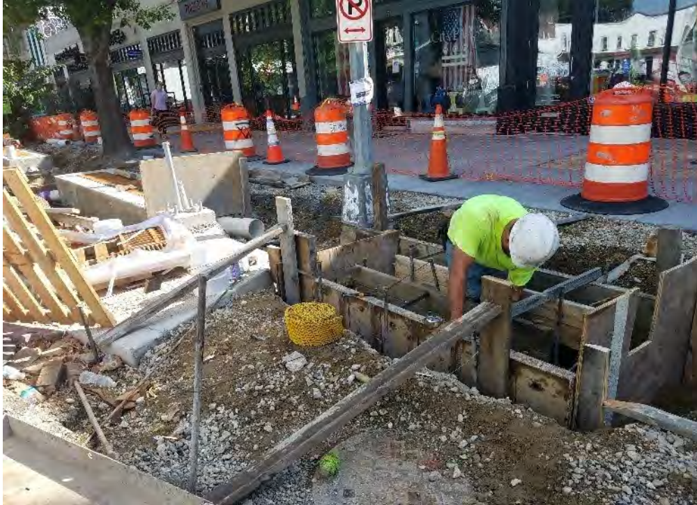
Modified section of trench added south of wheelchair ramp and pole foundation L80/PP
