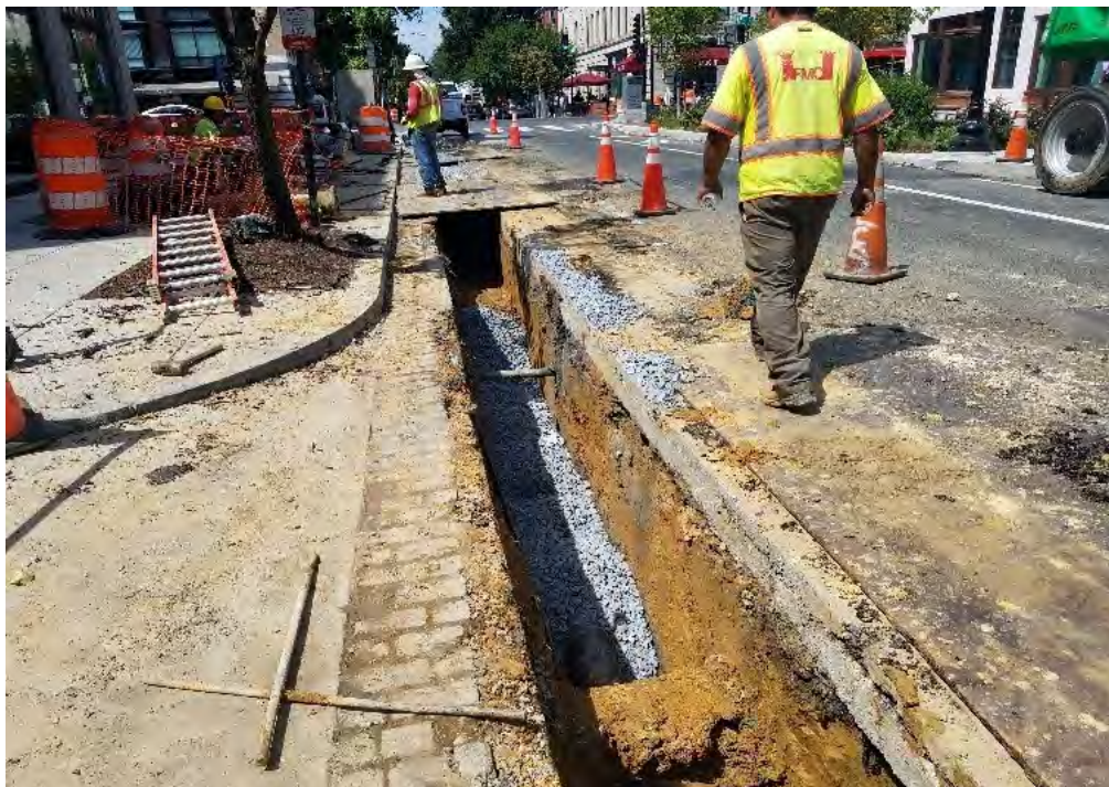
Omni working at westbound R St between 13 th & 14 th St placing 8" D.I.P.
