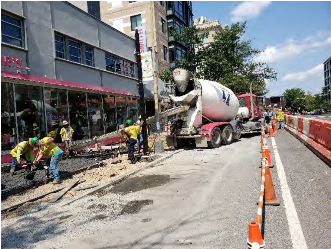
D.E.N. crew framed and poured one Building Ramp plus Sidewalk PCC near 14 th St. NW & R St. Intersection.
