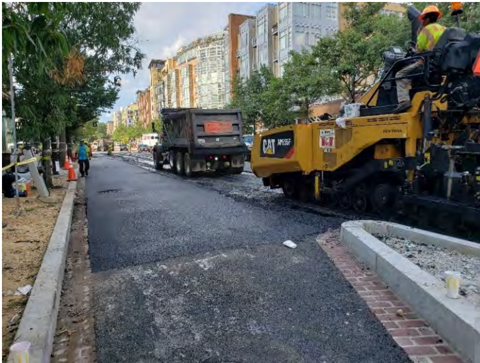
Surface Asphalt 12.5mm paving operation In-Progress at SB on 14 th St. near Bus Island at 2000 Block of 14 th St. NW.
