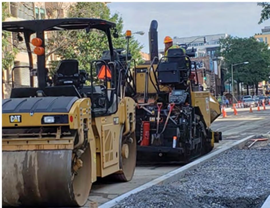
FMCC crew prepared Asphalt Paving Op by 9:30 am at NB 14 th St. NW.
