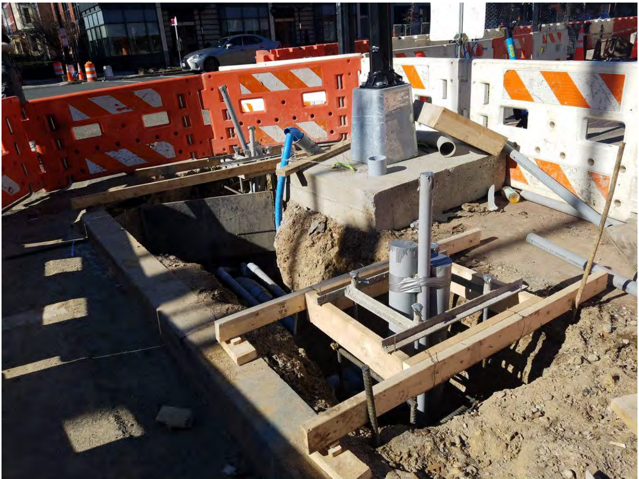
Traffic Signal Foundation at the NE Corner of 14 th and Q Street
