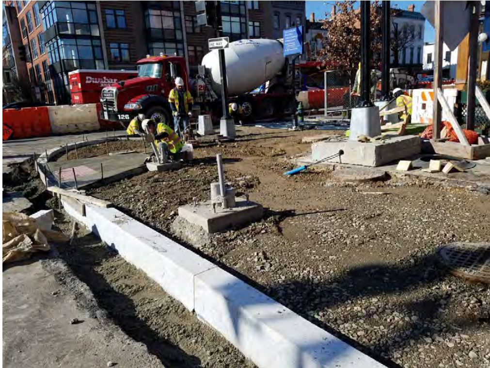
ADA Ramp placement at the NE Corner of 14 th and Q Street
