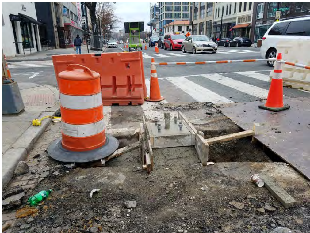
Street Light / Traffic Signal Foundation at the SW corner of Corcoran Street
