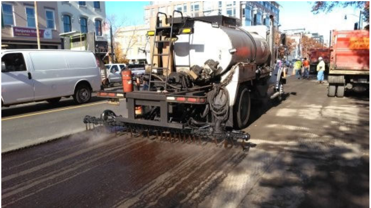
FMCC applying tack on the NB outside lane on 14 th Street NW between Riggs Street and S Street
