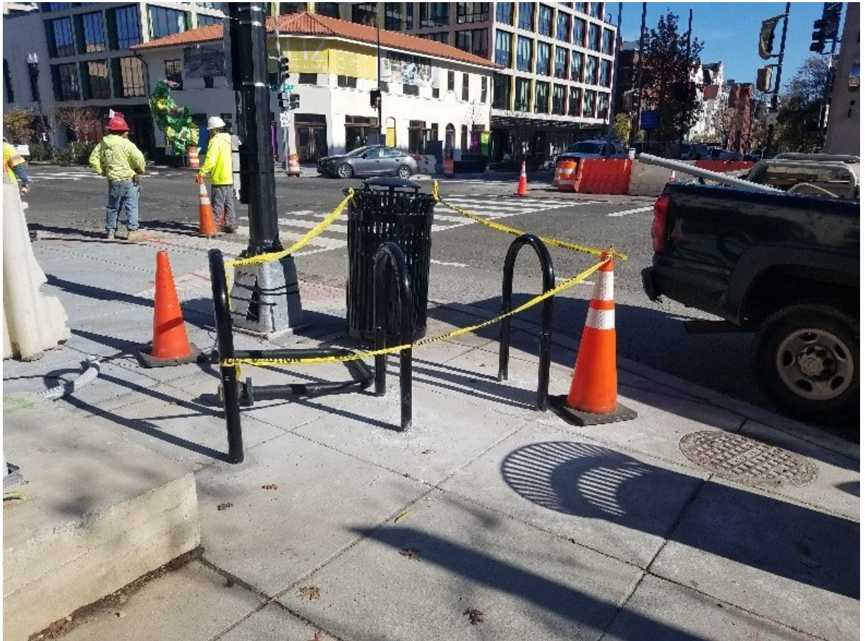
FMCC installing litter baskets and bike lockers at SWC of R St
