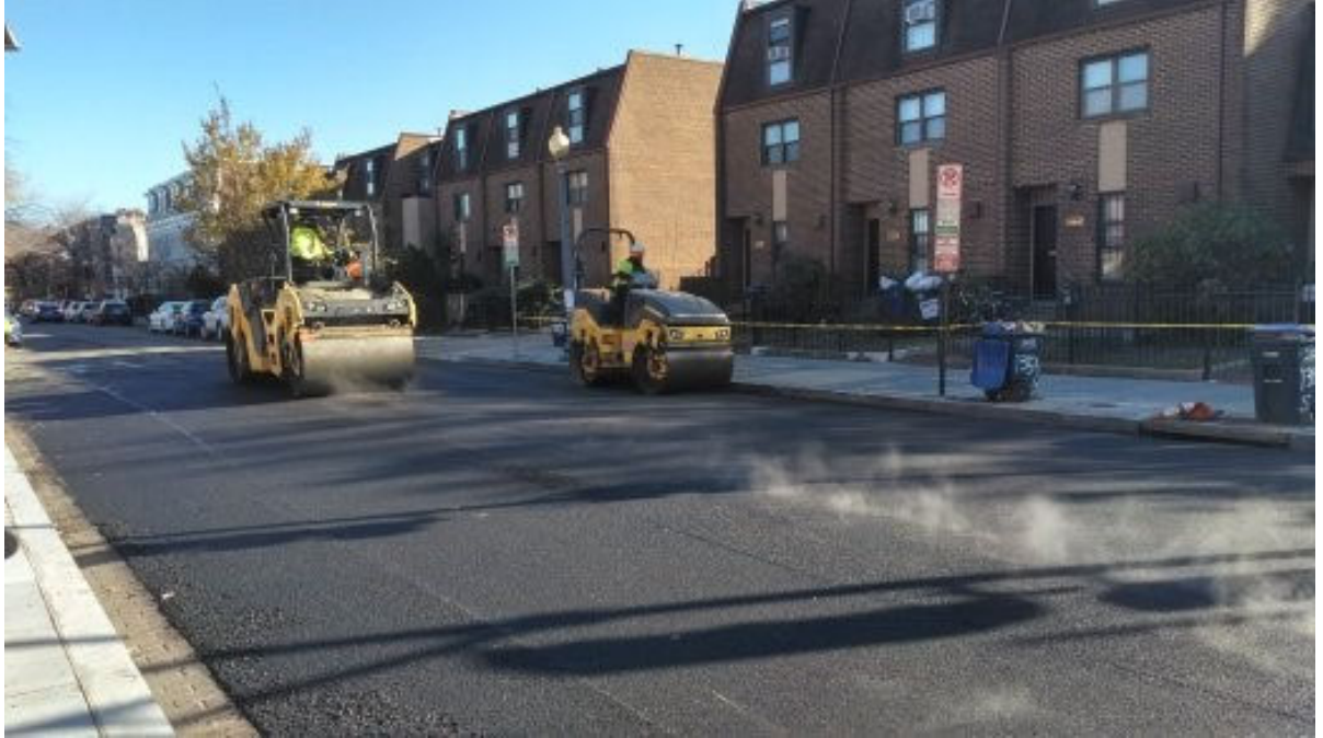
FMCC compacting the surface course 12.5 MM on S Street at NB 14th Street
