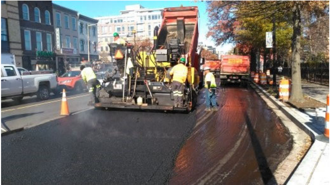
EFMCC paving the NB outside lane on 14 Street NW between Riggs Street and S Street
