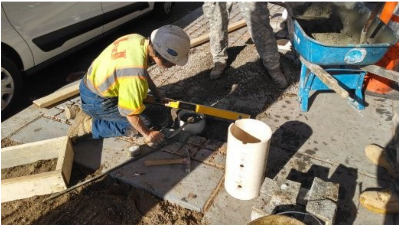
Installing bench foundations between U street and V street on 14 th Street NW
