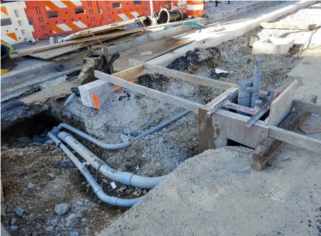
2" & 4" PVC conduit shown at NWC of 14 th St at TS-27 & Hand box HB-09
