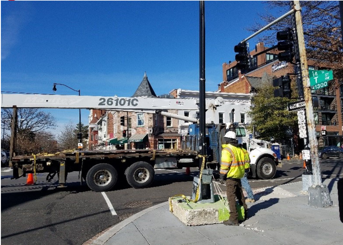
Loading of temporary bases by FMCC at NEC of 14 th & T St.
