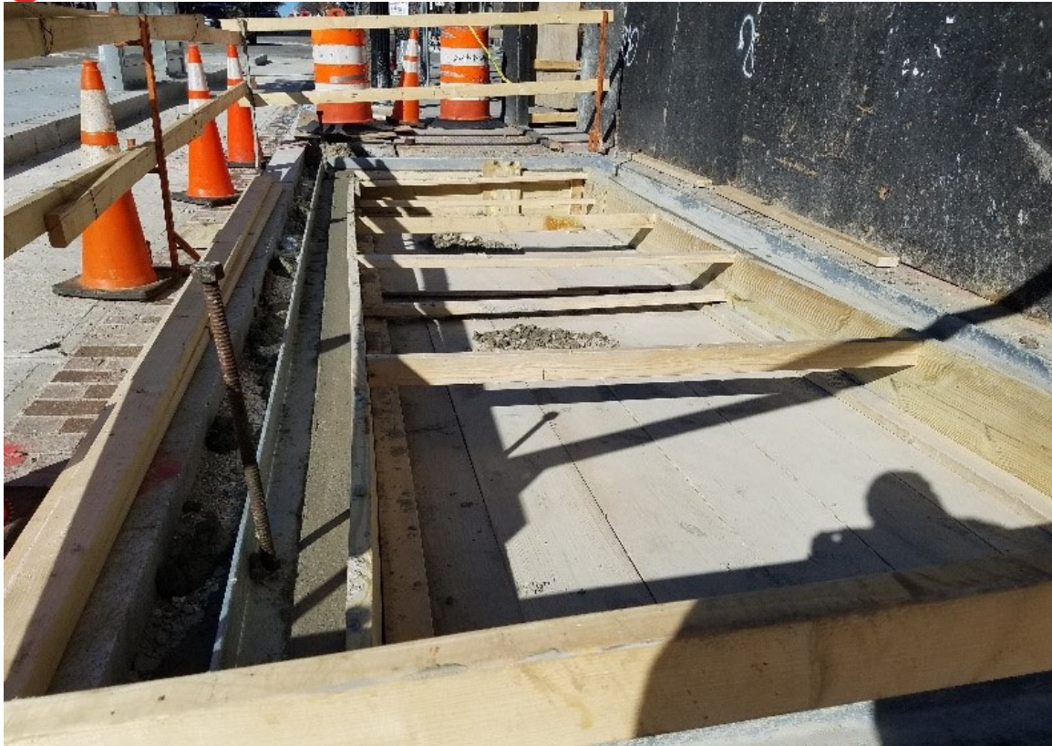
Pepco vault at 2200 block of 14 th St near Ellisdale project framed and concrete placed
