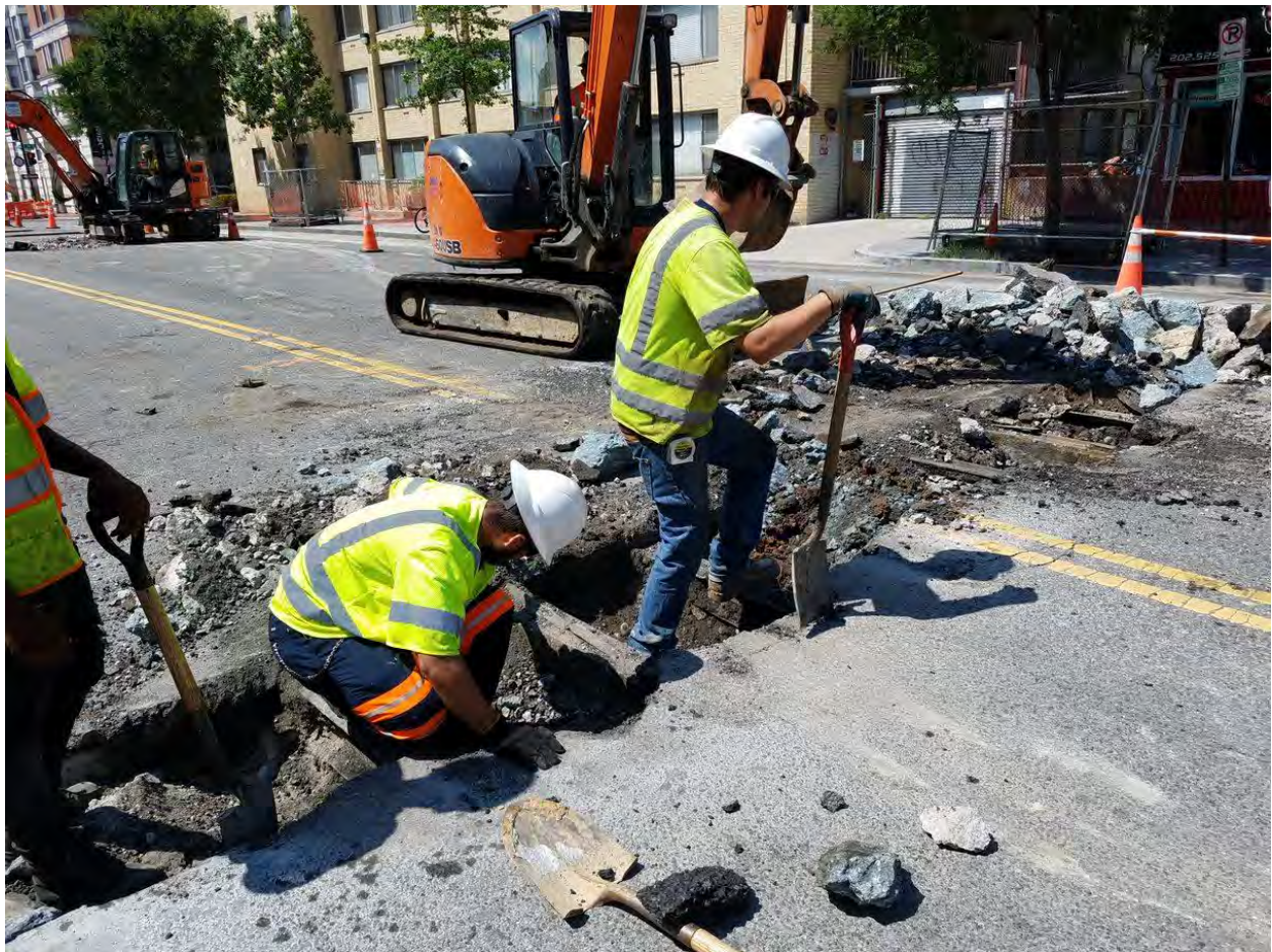
Excavation for the Laterals between N Street and Rhode Island Ave on the Westside
