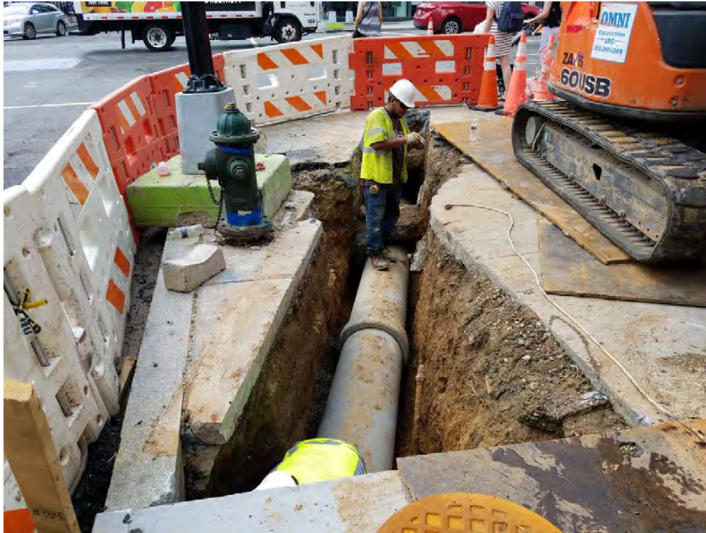
Installation of Catch Basin 15" PCC Connection pipe at NE corner of 14 th and P Street
