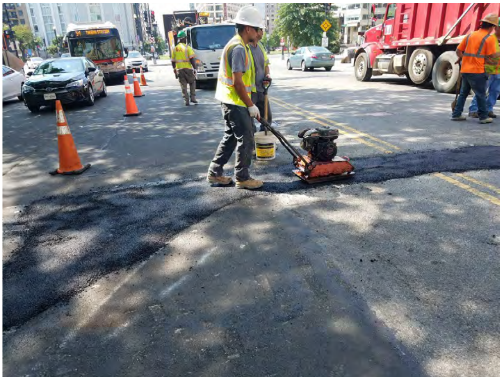
Placement of Temporary Asphalt over Laterals between Thomas Circle and N Street
