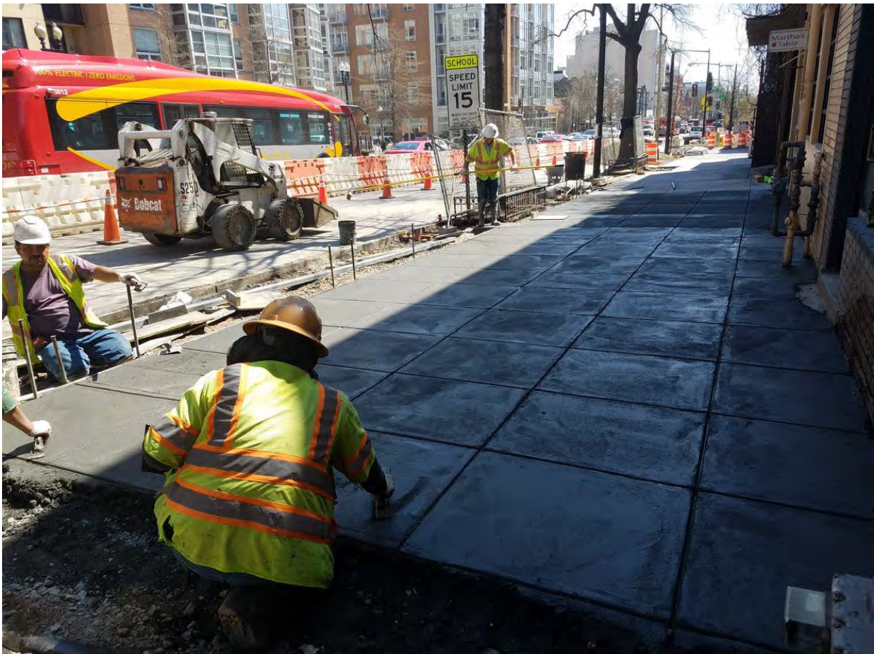
Installation of New PCC Sidewalk between V and W Street on the Westside
