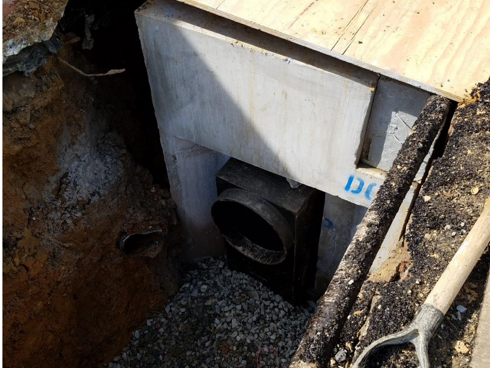
Installation of Water Seal into the Catch Basin before 15" PCC Connection pipe is installed
