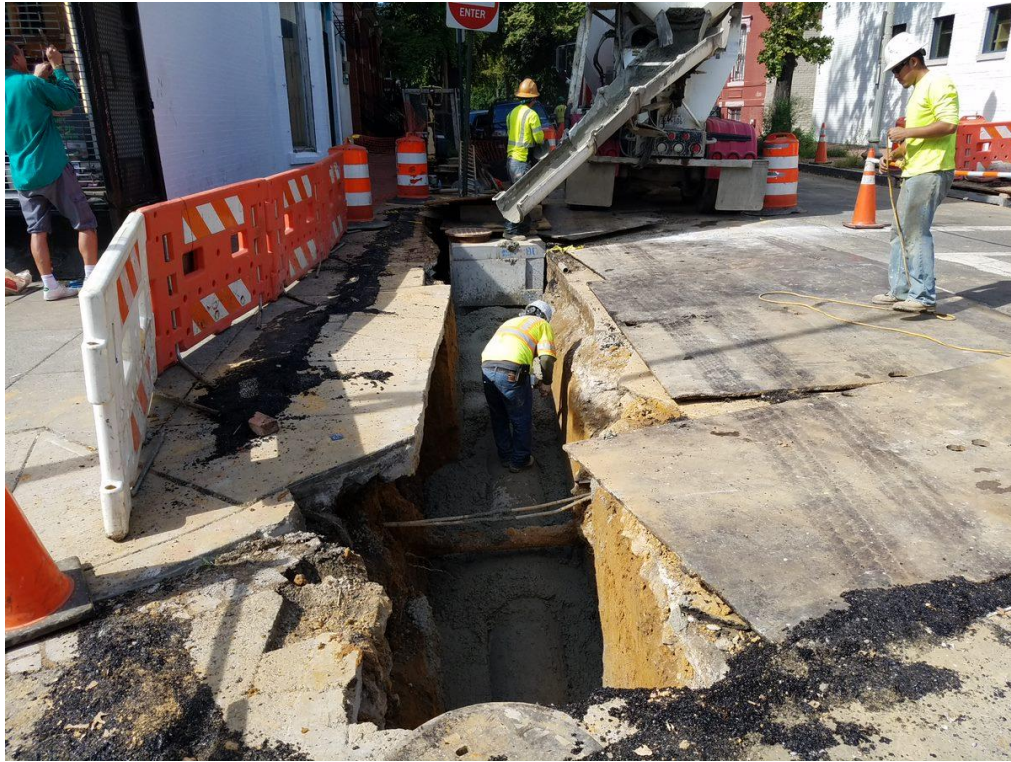
Pouring DC Wasa Mix for the Cradle for the 15" PCC Connection Pipe
