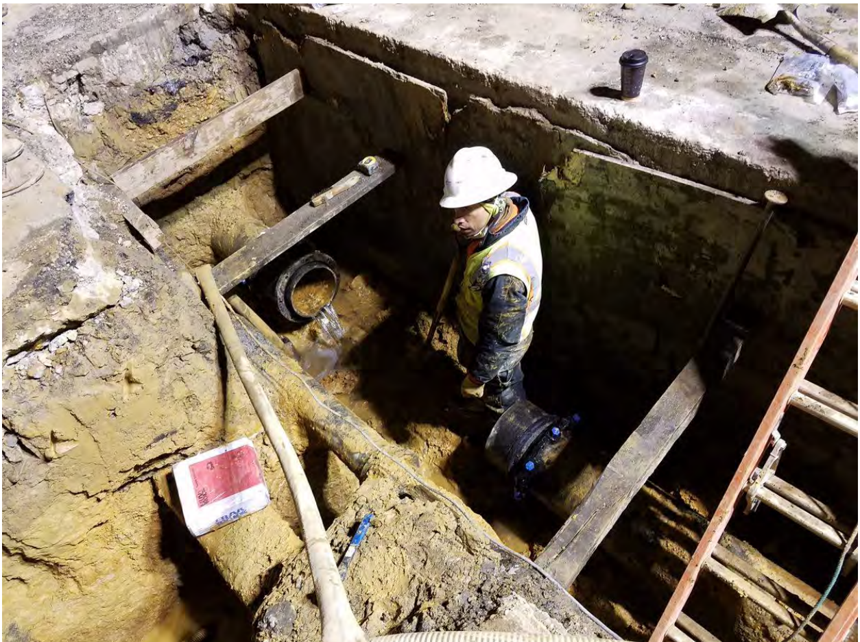
Installation of New Fire Hydrant at 14 th and Church on the Westside
