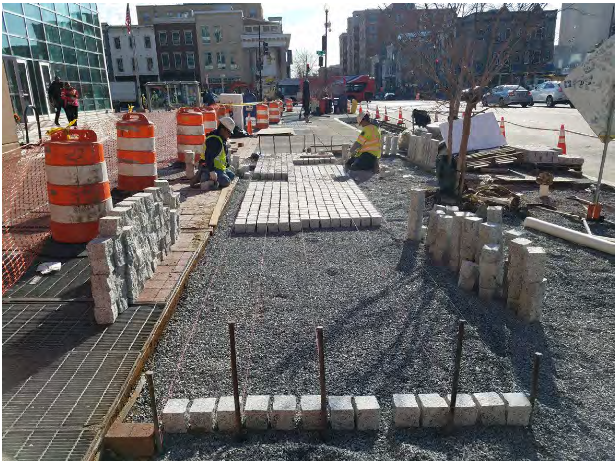
Installation of Granite Cobble Stone around Tree Box Area on U Street
