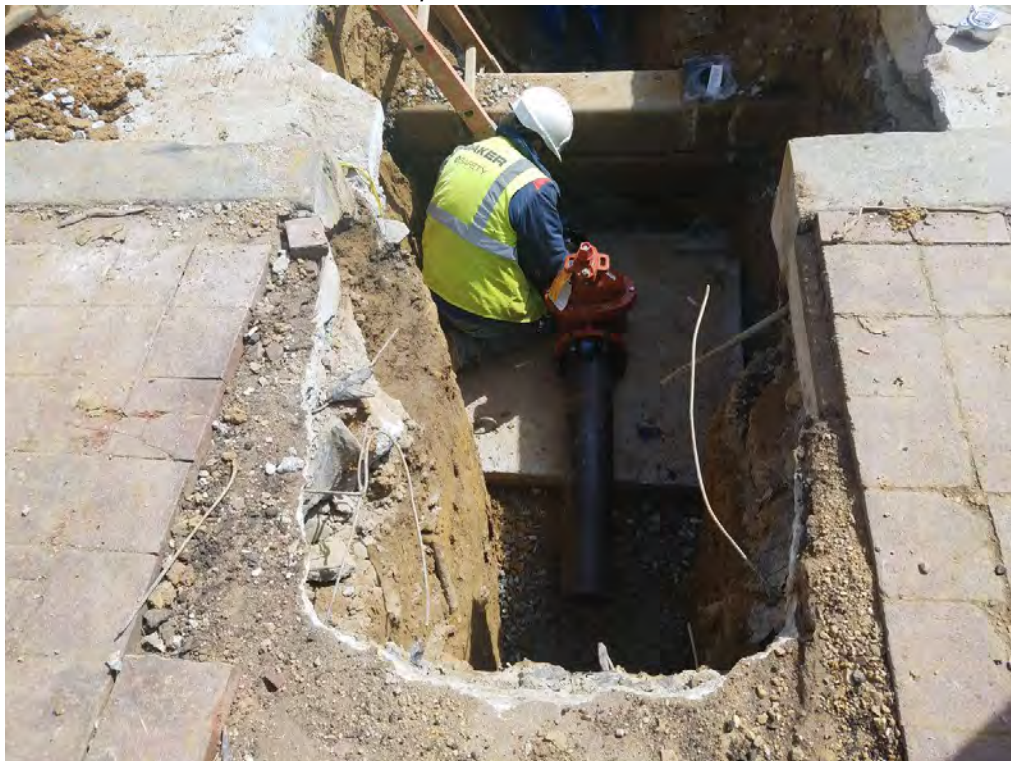
Installation of Gate Valve for New Fire Hydrant at 14 th and U Street
