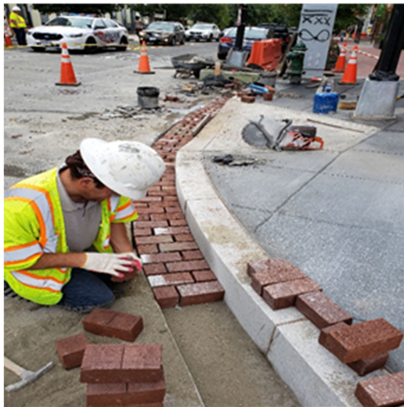
DEN placed Brick Gutter and Granite at 1350 Florida Ave. at Crosswalk at 14 th St. NW Intersection. But, DEN Saw Cut PCC base by 6" beyond the 12" Brick Gutter & It will be fixed later & it falls within Bus Island Zone.
