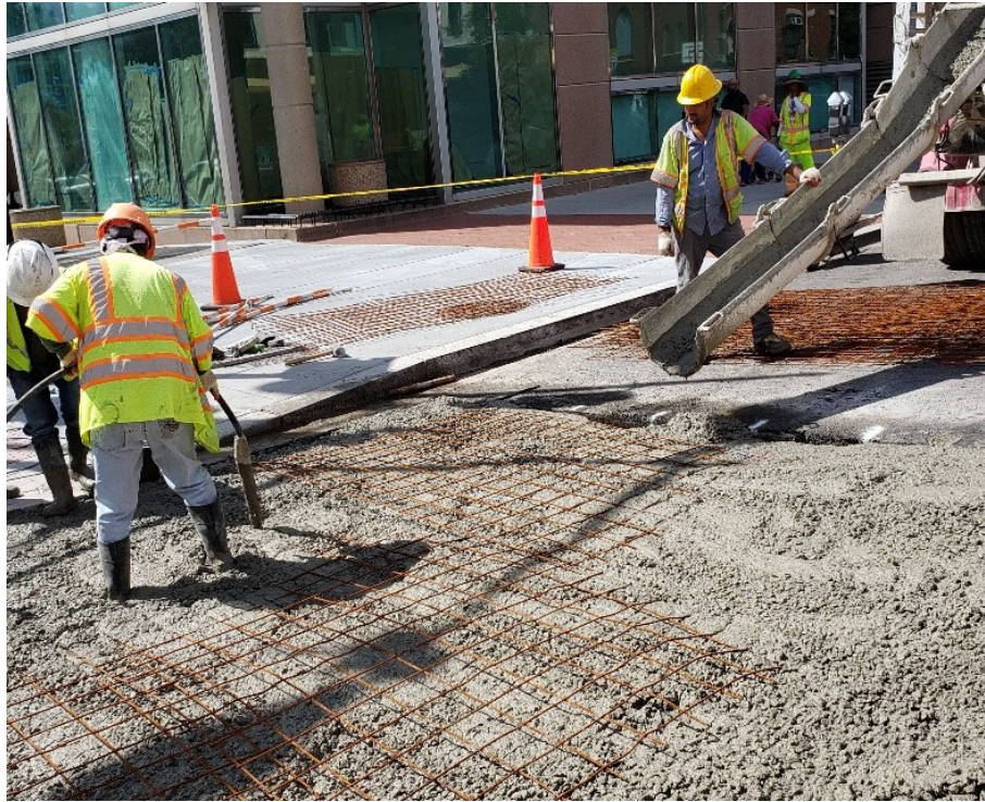
D.E.N crew poured PCC 10" Class E with Roadway Dowels drilled into PCC Base & Wire Mesh at V St. NW & 14 th St. Intersection.
