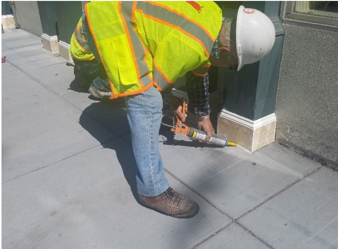
Wood molding sealed by FMCC
