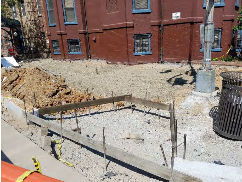
Placing of Structural Soil at the NE corner of N Street Eastside
