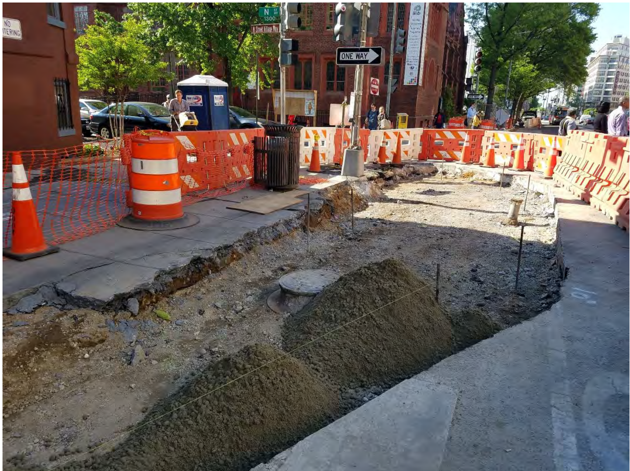
Installation of Bump Out at the NE corner of N Street on the Eastside
