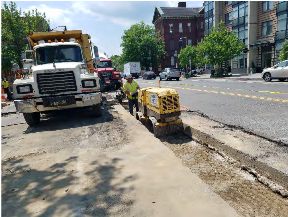
Compaction of Backfill over encased PVC Conduit between P and Q Street
