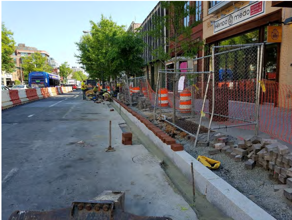
Placement of Brick Gutter between N Street and Rhode Island Ave Eastside
