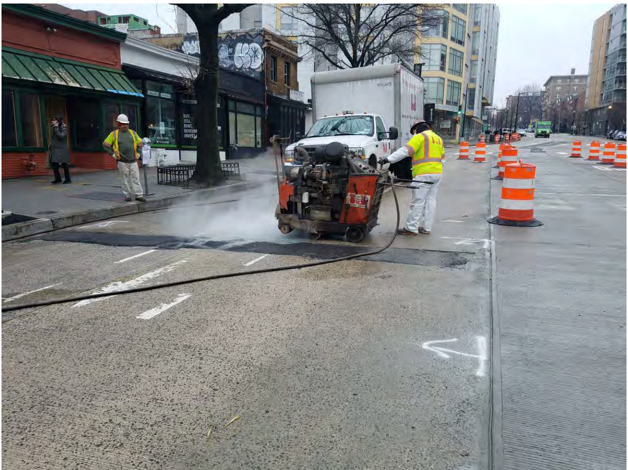
Saw Cutting for PCC Pavement Repair between Florida Ave and W Street
