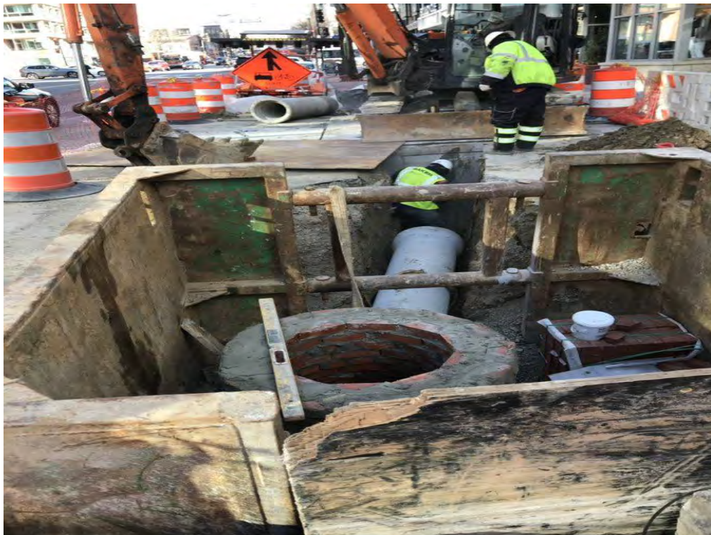
Installation 15" PCC Connect Pipe into Brick Sewer Manhole at 14 th and Wallach
