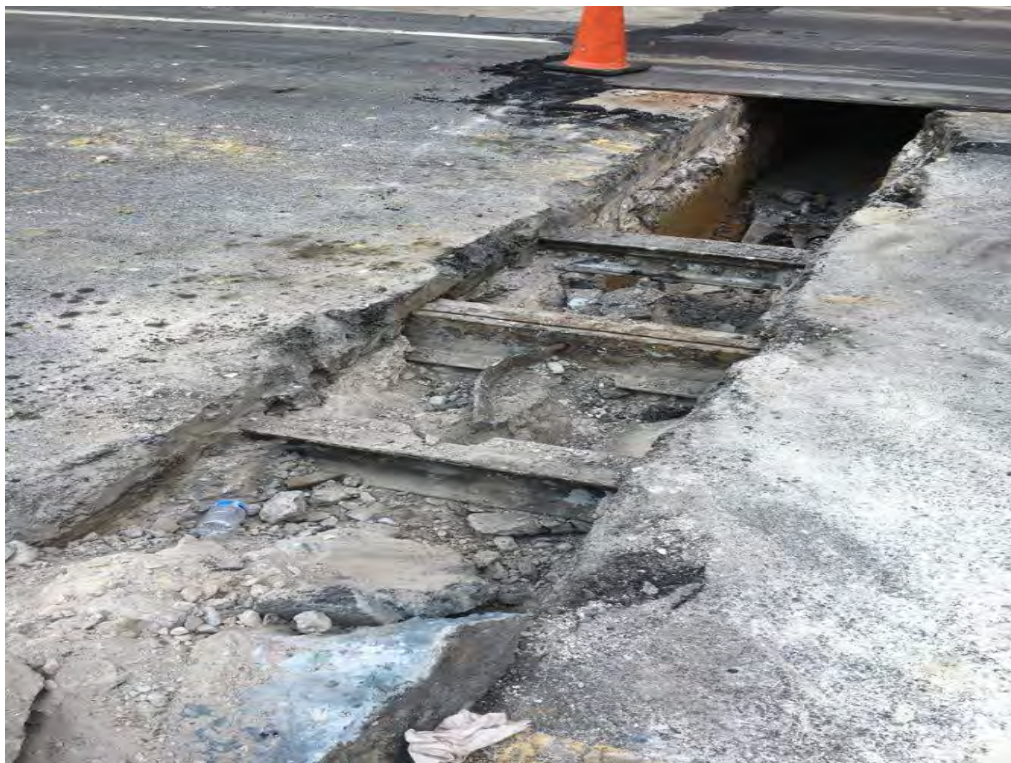
Abandon Street Car Track to be removed
