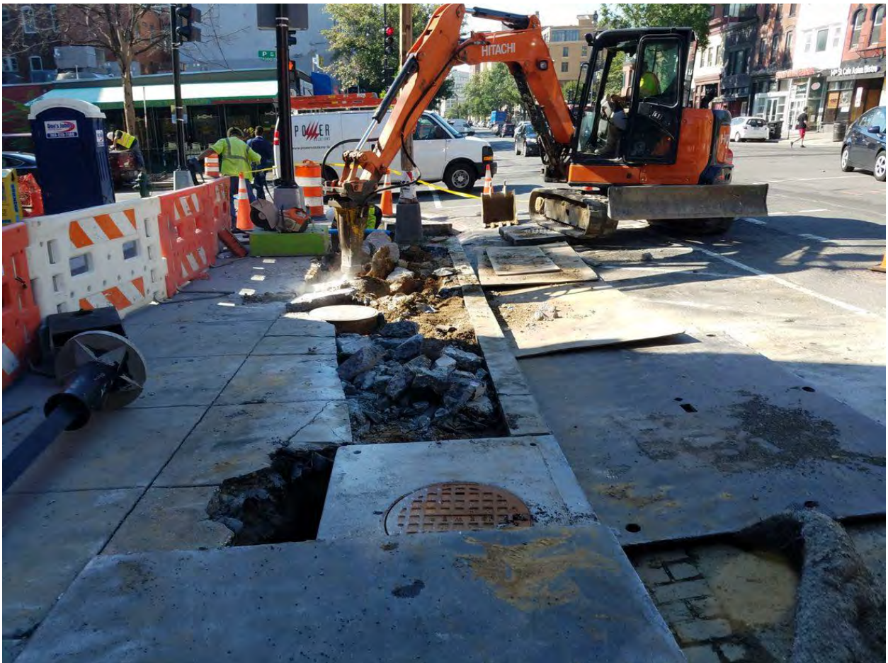
Excavation for the Connection pipe to Double Catch Basin at NEC of 14 th and P Street
