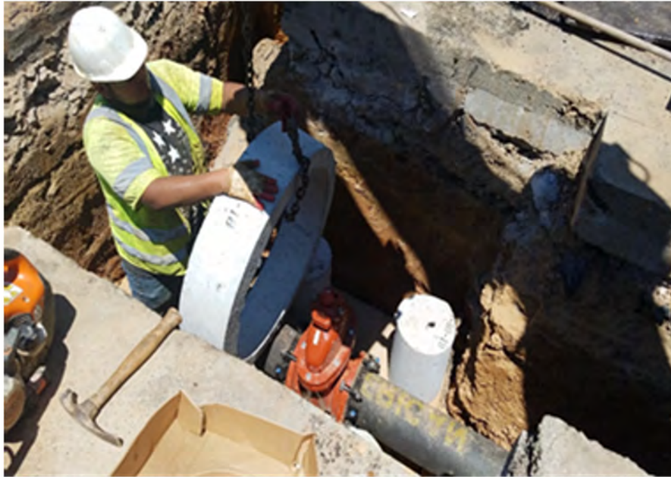
8" gate valve and casing installed by Omni
