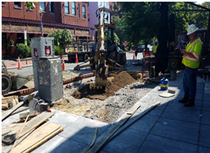
Tree zone at SEC of 14 th & T St with structural soil placed.
