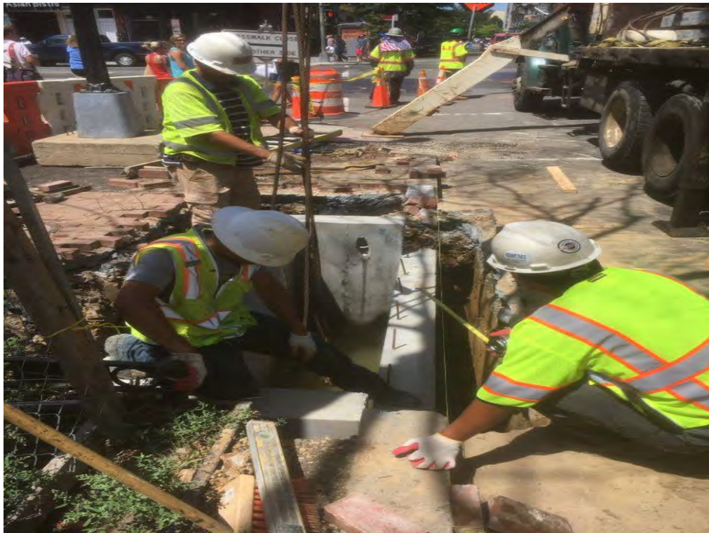
Installation of the Double Catch Basin on SE Corner of P Street
