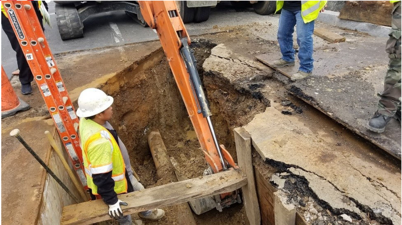
Omni was noticed working without proper trenching at T Street
