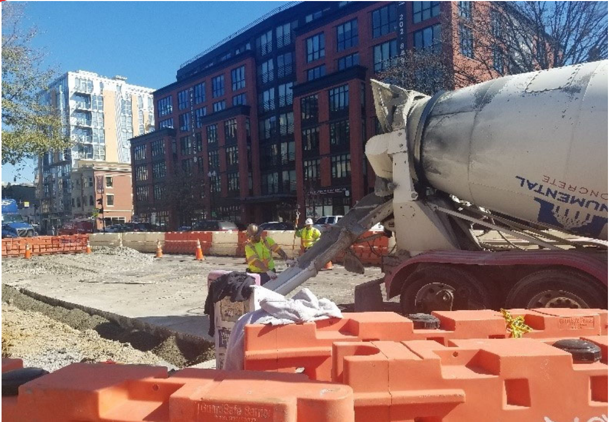
Class F dry mix placed by D.E.N. for granite curb placement at NWC of 14 th & T St
