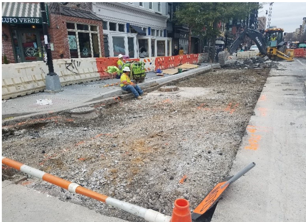
FMCC civil crew excavating roadway for future directional bus island at NWC of 14 th & T St
