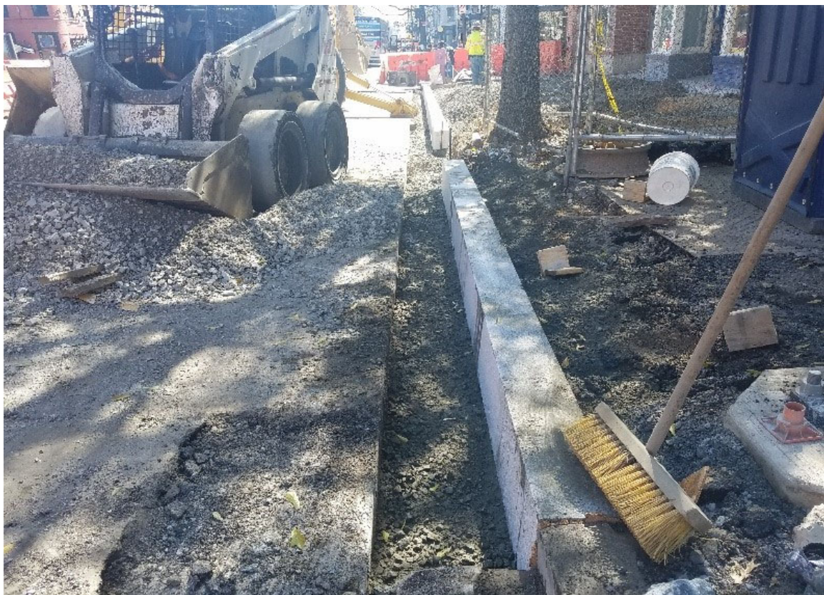
Straight granite curb placed at NWC of 14 th & T to 1908 14 th St.
