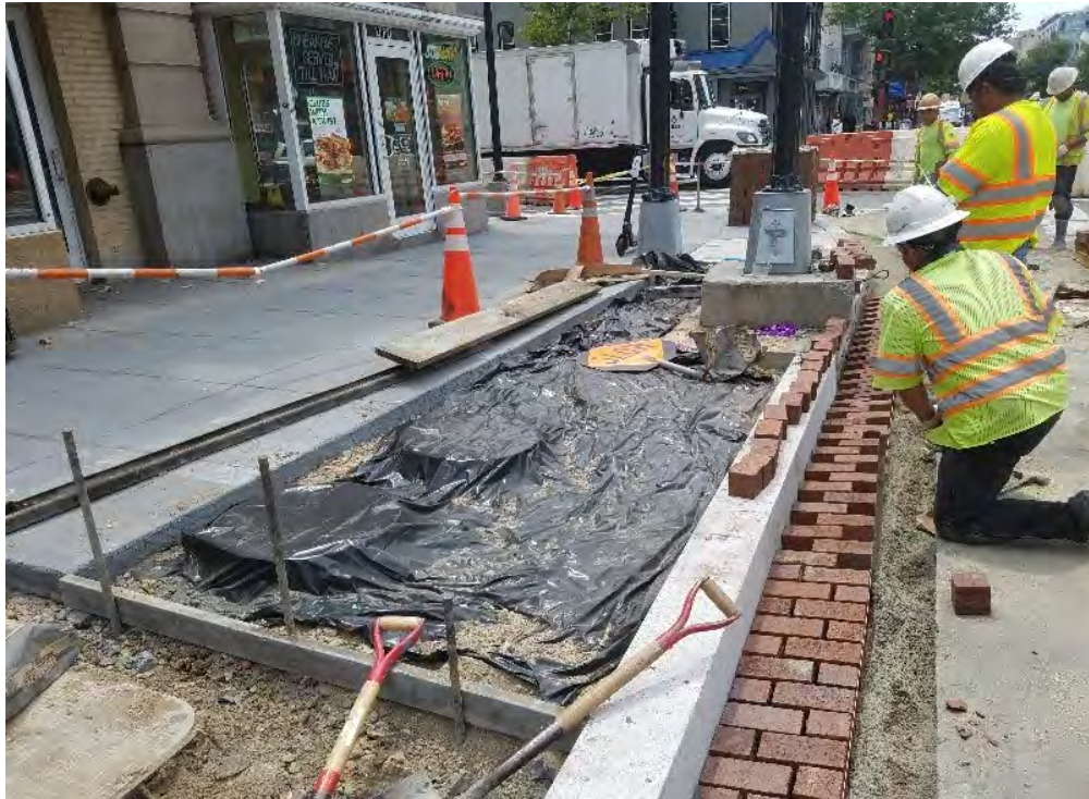
Brick gutter placement and sidewalk section ready for placement at NEC of 14 th & U St.
