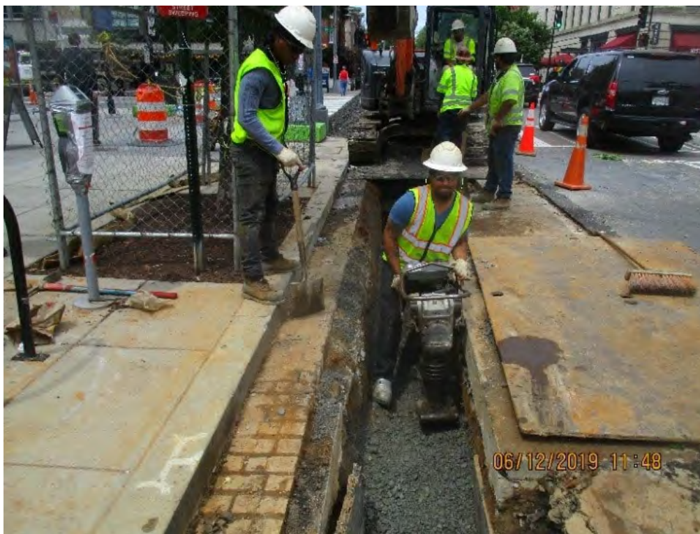
Omni compacting the backfill material in the trench excavated for the installation of 8-Inch D.I.P at R Street NW
