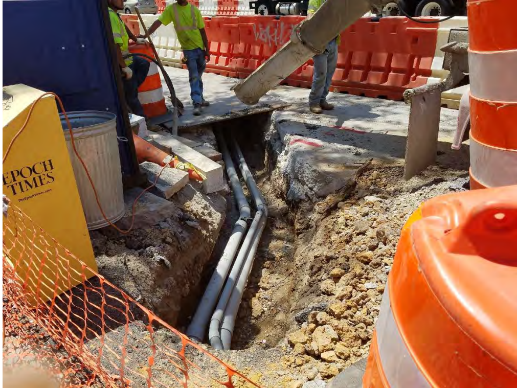
Installation of PVC conduit to the Bus Island Location at N Street
