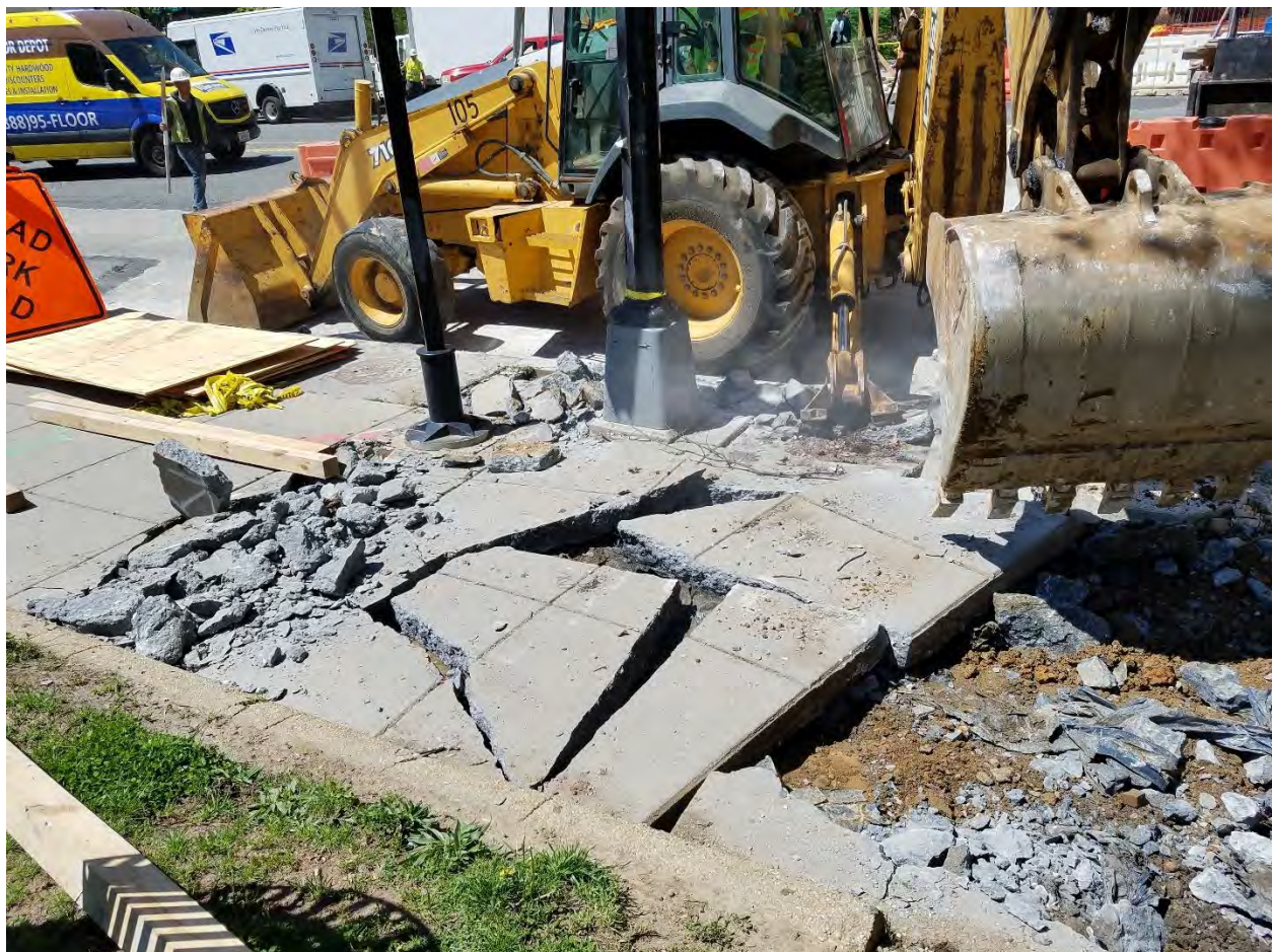
Demo of Existing Sidewalk between Thomas Circle and N Street on the Eastside
