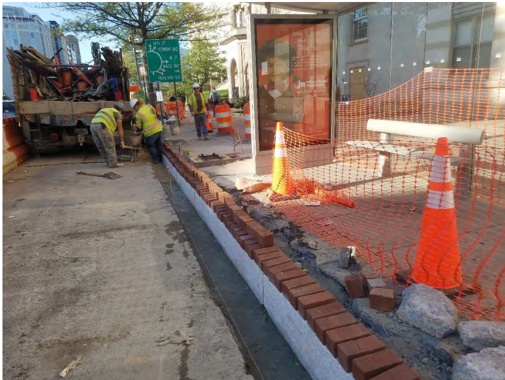
Placing of Granite Curb and Brick Gutter N Street to Thomas Circle Westside
