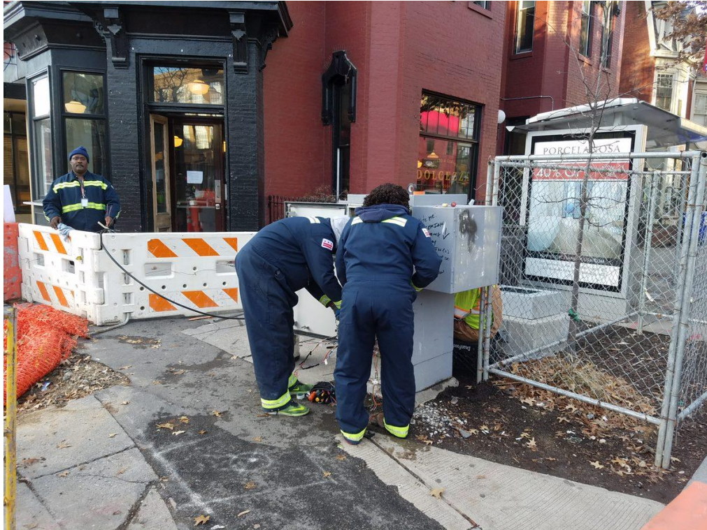
DDOT Technician working on the Traffic Control Cabinet for the relocation at SW corner of P Street
