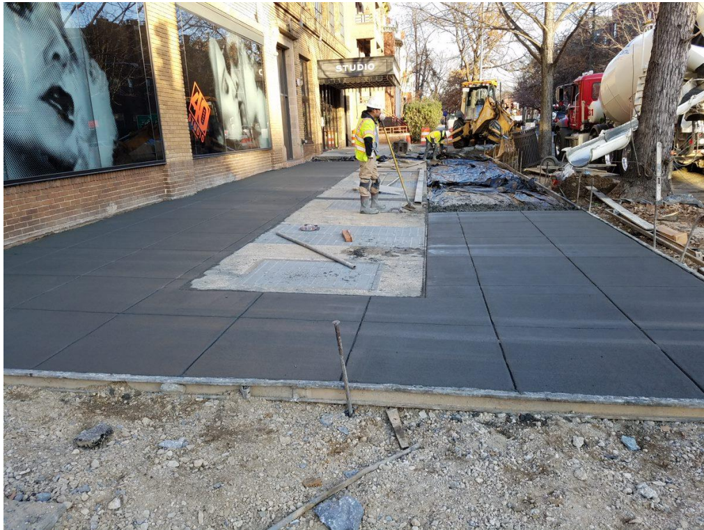
Placement of PCC Sidewalk at the NE Corner of 14 th and P Street
