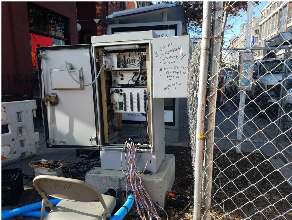
Traffic Control Cabinet on Temporary Base at the SW Corner of P Street
