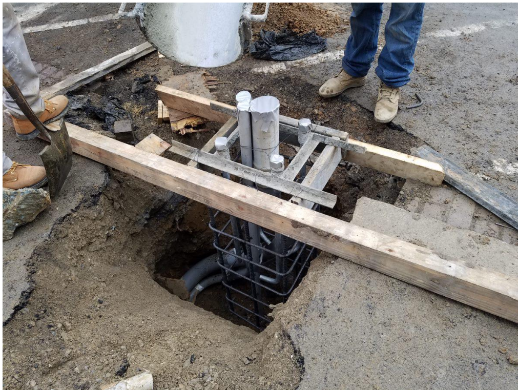
Forming of the Traffic Signal Foundation at the NE corner of P Street
