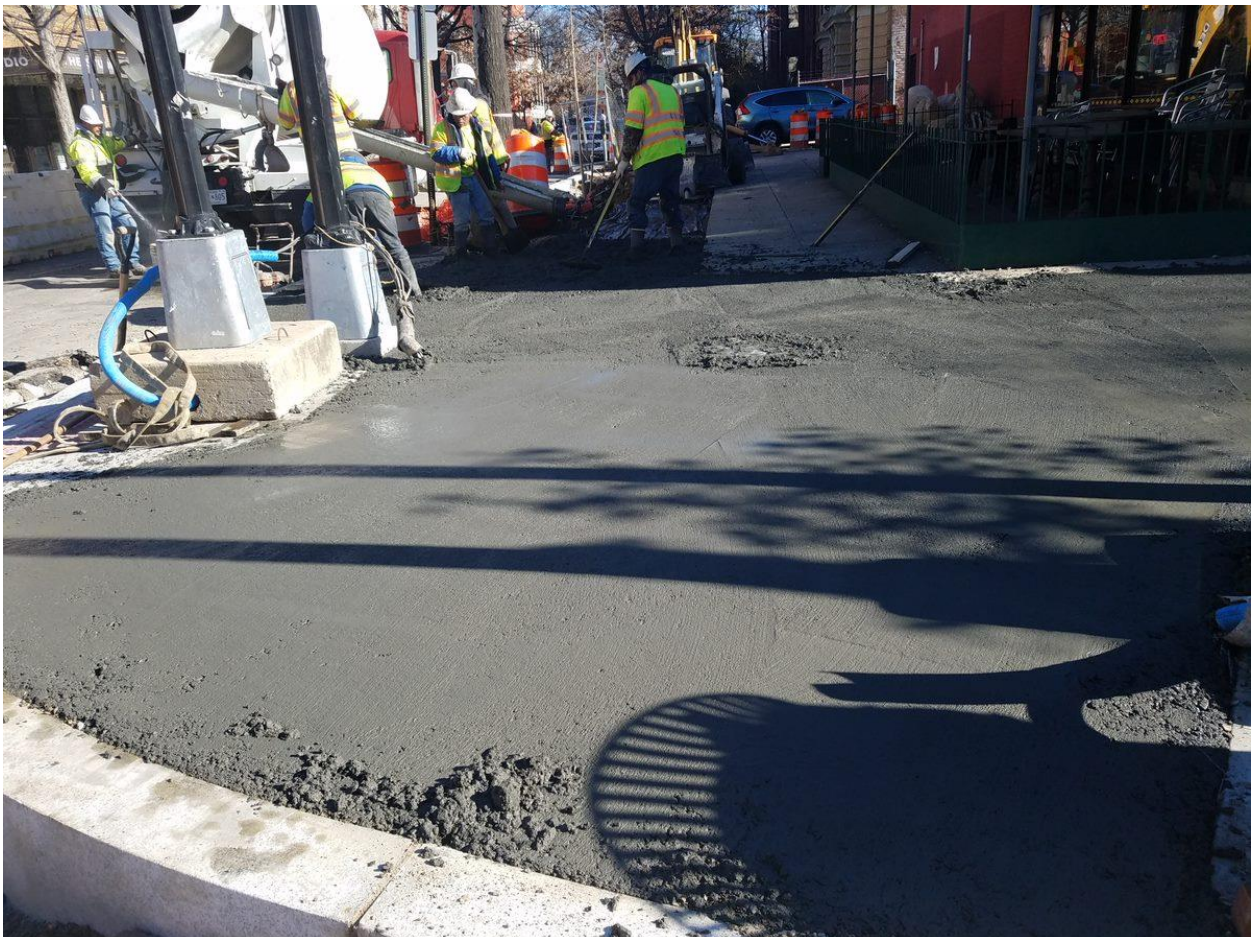
Placement of PCC Sidewalk at the SE Corner of 14 th and P Street
