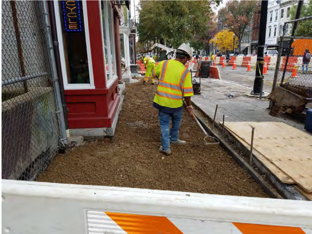
Aggregate Base Material placement prior to PCC Sidewalk between N Street and Rhode Island Ave
