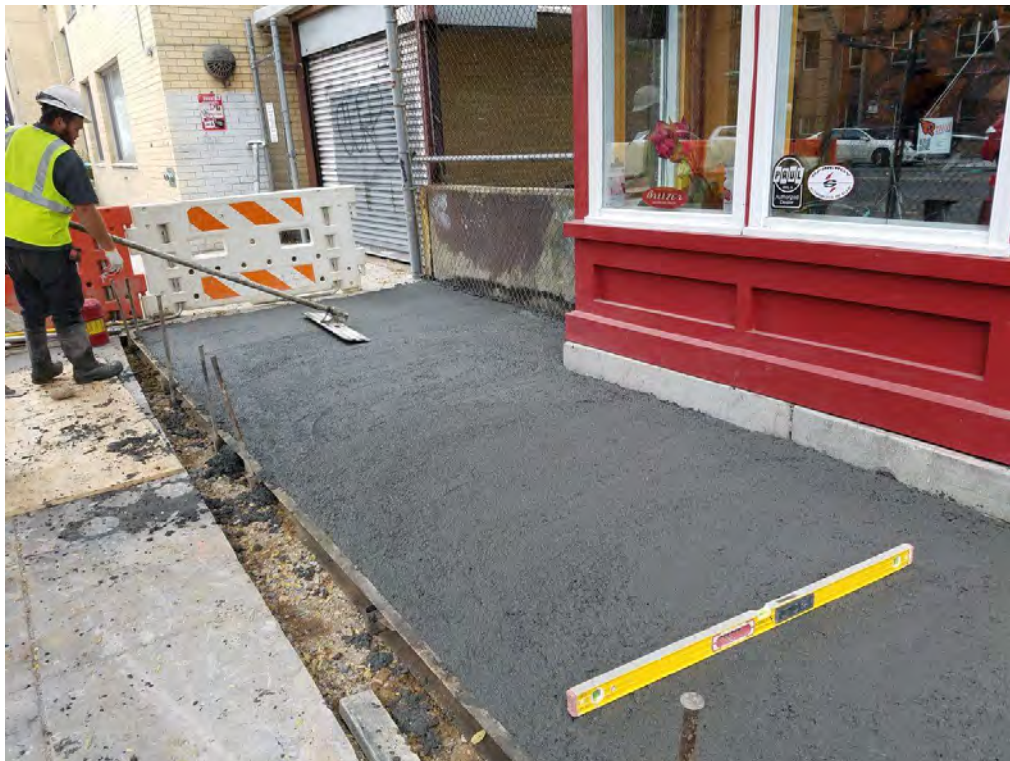
PCC Sidewalk Replacement between N Street and Rhode Island Ave on Westside
