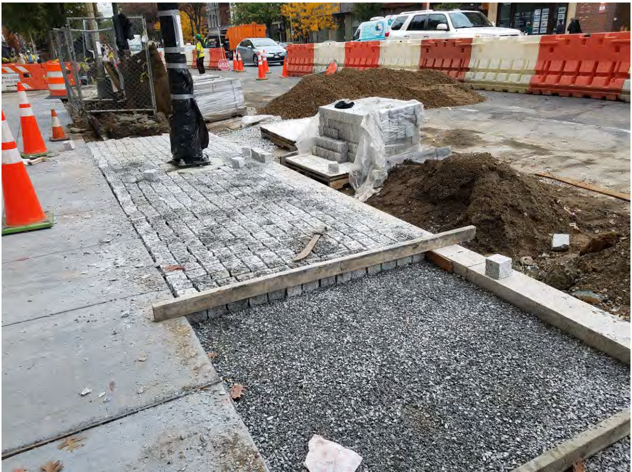
Installation of Permeable Pavers (Granite Cobble Stone) between N Street and Rhode Island Ave
