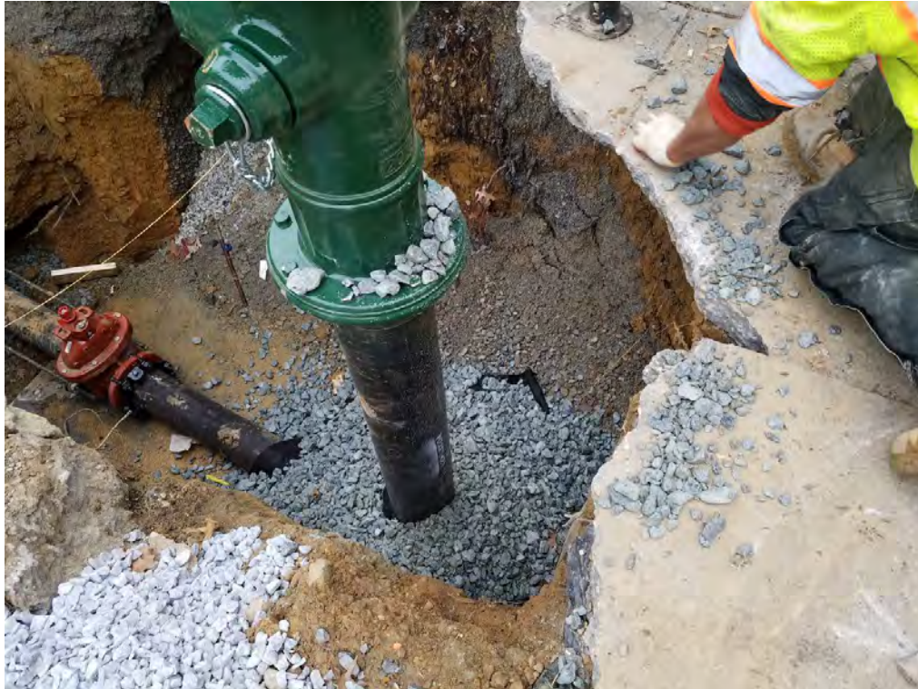
Installation of New Fire Hydrant at the NE corner of 14 th and Q Street
