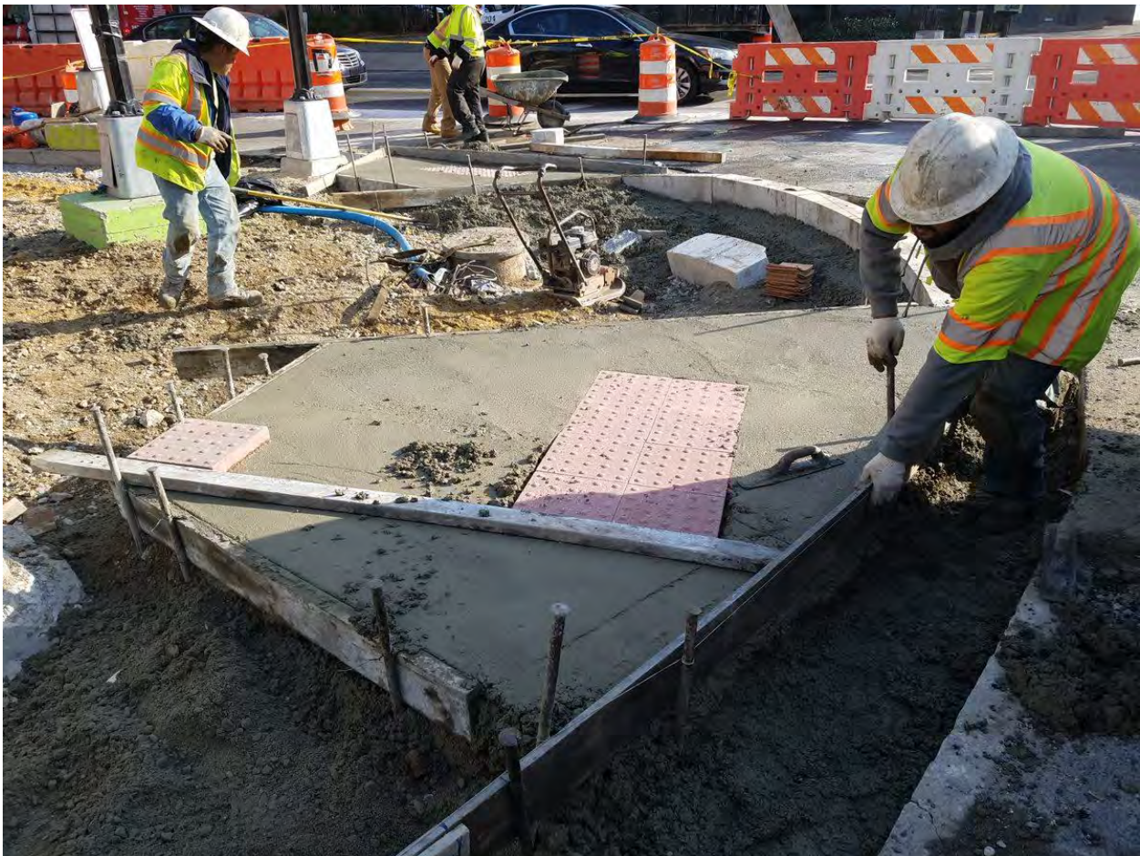
Placement of ADA Ramps at the NE Corner of 14 th and Rhode Island Ave
