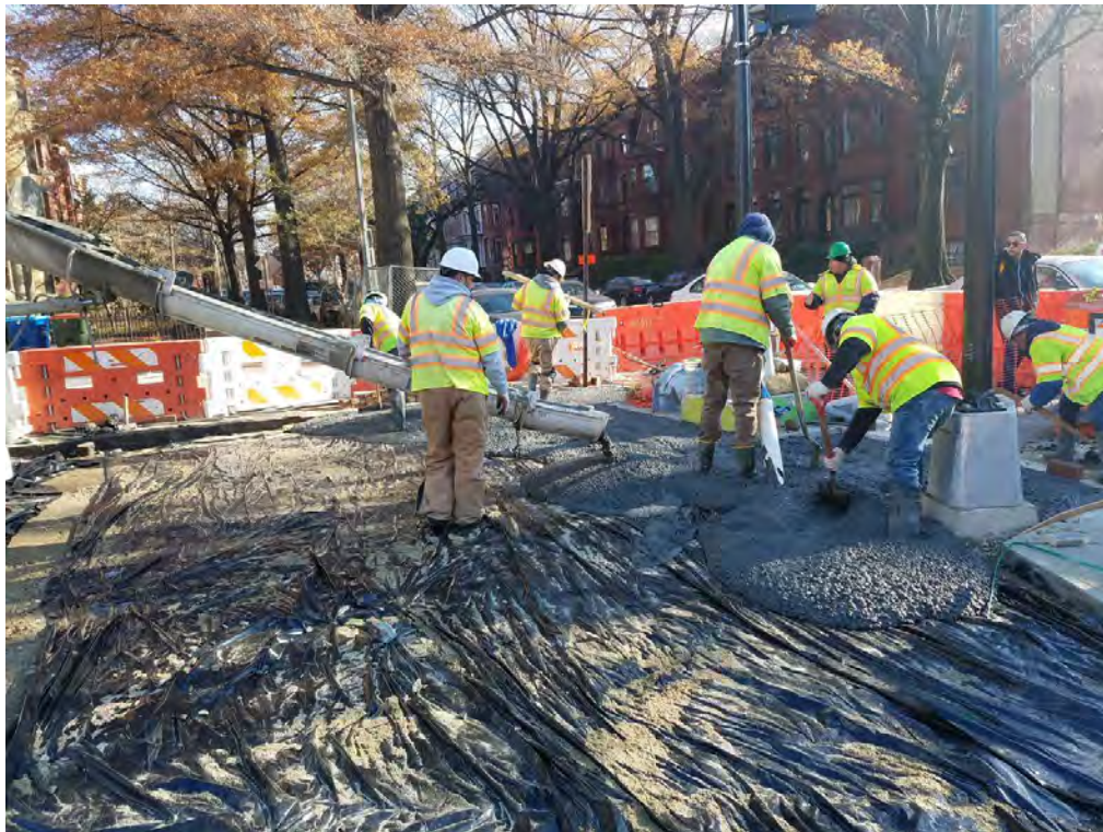
Placing PCC Sidewalk at the NE Corner of 14 th and Rhode Island Ave
