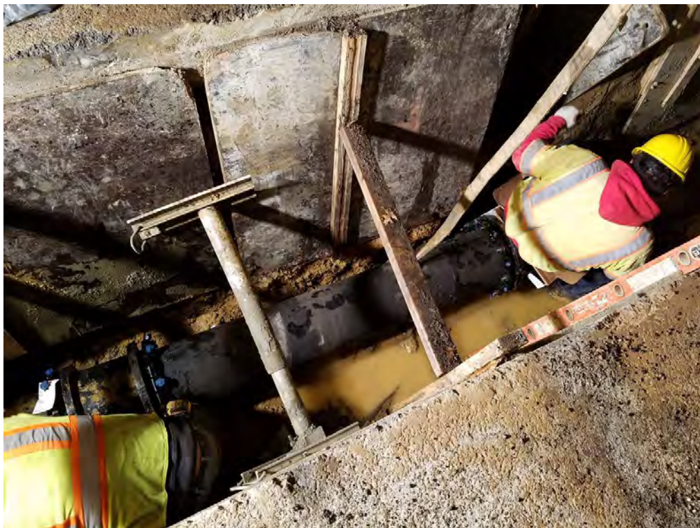
Installation of a new piece of 12" Water Main Pipe at 14 th and Q Street
