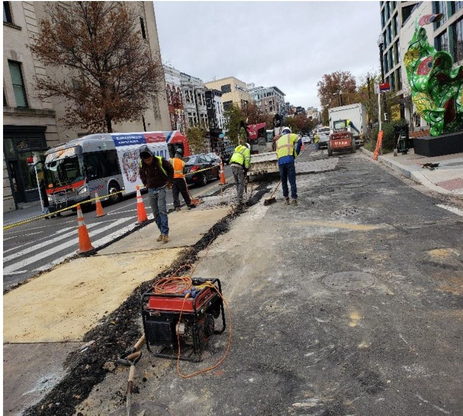
OMNI, Inc. secured and Welded total Ten (10) Steel Plates on Saturday, 11-9-2019 at Intersection of R St. & 14 th covering the Traffic Signal Trench NB.
