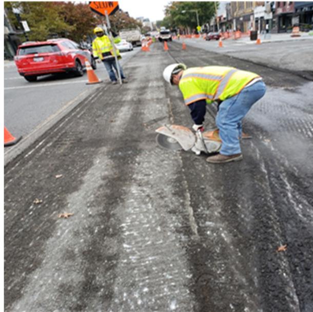
FMCC Asphalt crew also saw cut the exposed portion of Old Track Metal Railing eliminating a potential Roadway Hazardous condition, on Thursday, 11-7-2019.
