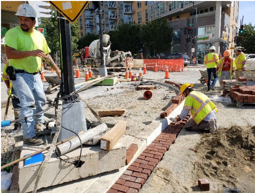
DEN crew also placed Brick Gutter at SWC of Near 2300 Block 14 th St. NW.
