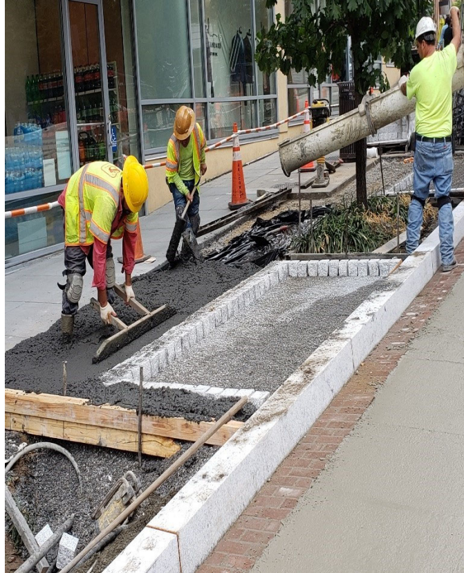
DEN placed 4" GAB, and PCC Sidewalk next to Permeable Stone and Tree Boxes at 14 th St. & FL Ave.
