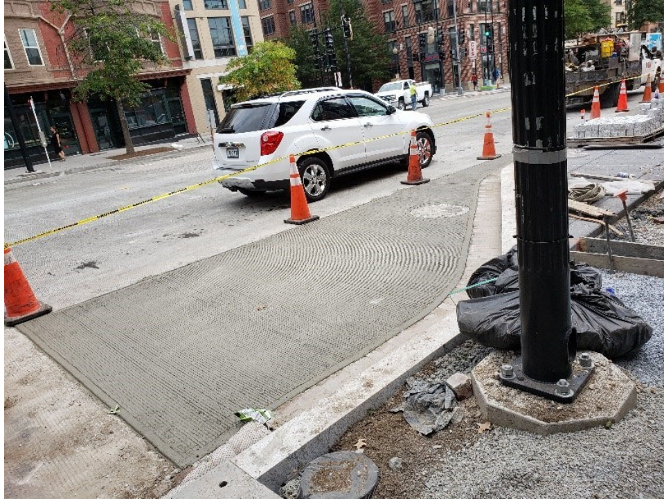
D.E.N. excavated the Bump-out area & placed PCC-Base 10" Class E with Mesh-Wire & Dowels at 14 th St. NW.
