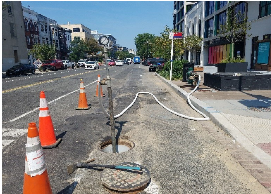
Pressure test gauge connected to standpipe at NB 14 th St
