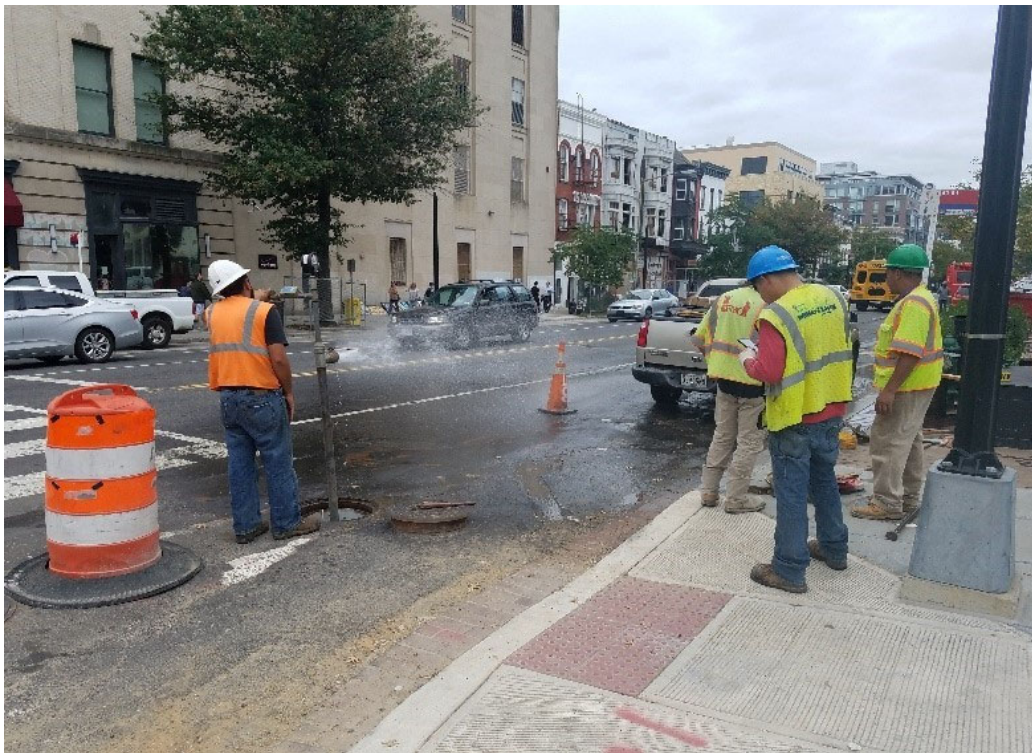
Stand pipe valve at northbound 14 th St connected to pressure gauge.
