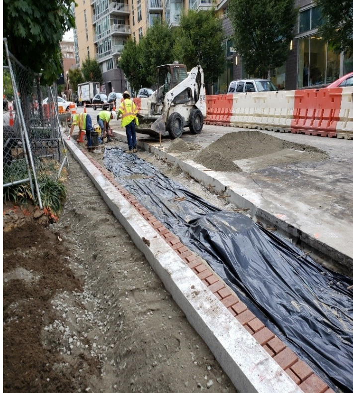
DEN Crew placed PCC-Base 10" section poured ranged in width between 3 Ft and 7 Ft.; at 14 th St. NW.
