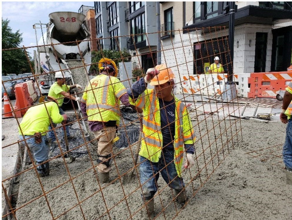
D.E.N crew excavated; then placed PCC Base 18 Cubic Yards, Class E Near 1405 W St. & 14 th St. NW.
