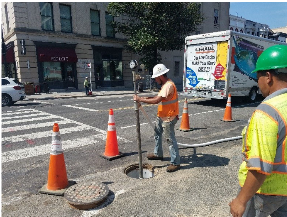
Pressure test incomplete due to defective test gauge.
