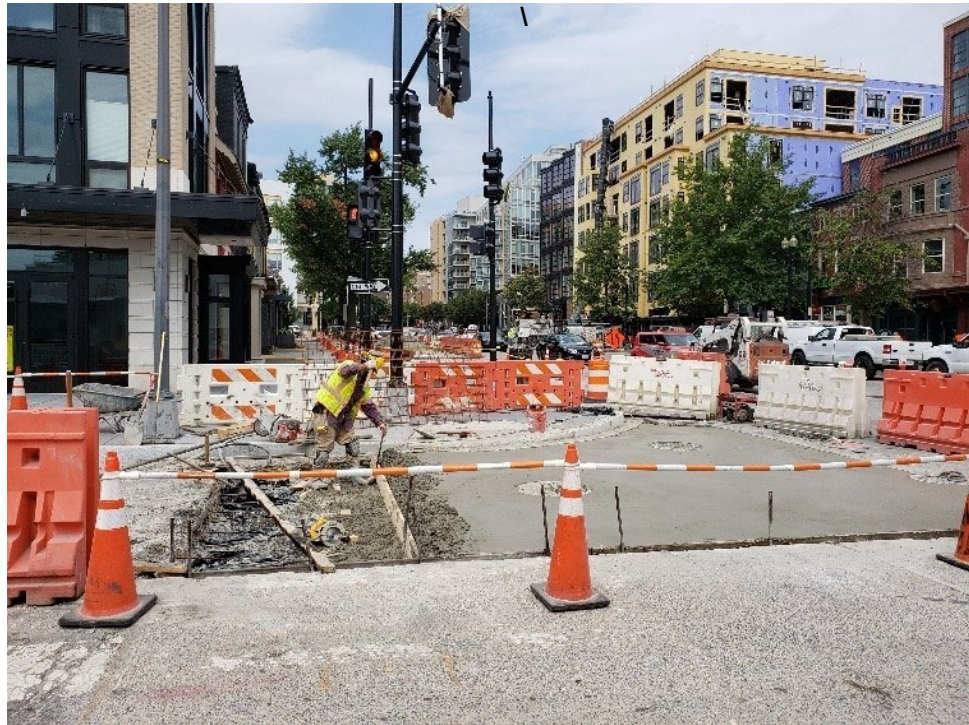
DEN Placed 18 C.Y. PCC Base 10" at SWC of 14 th St. NW & W St. NW Intersection on Mon 9-9-2019.
