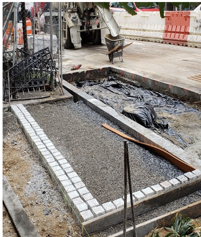
DEN Crew placed GAB 6" in Depth for PCC 10" plus vapor barriers and Dowels at 14 th St. NW & Florida Ave.
