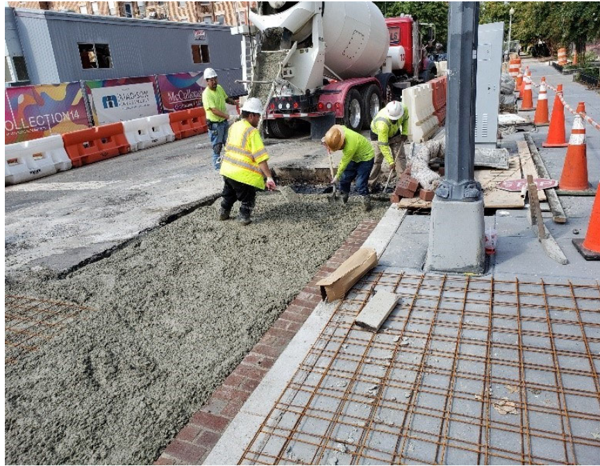
DEN Crew placed Roadway dowels drilled into existing PCC Base along with WWF (Wire-Mesh) for Reinforcing of PCC 10" Base.
