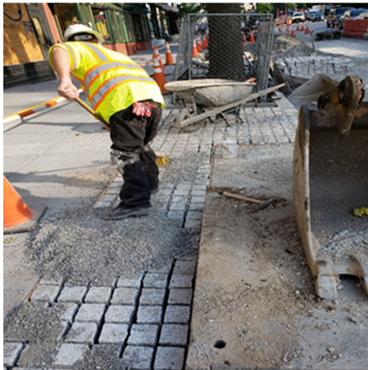
DEN Crew installed Permeable Cobble Stone next Sidewalk topped off with # 8 materials.
