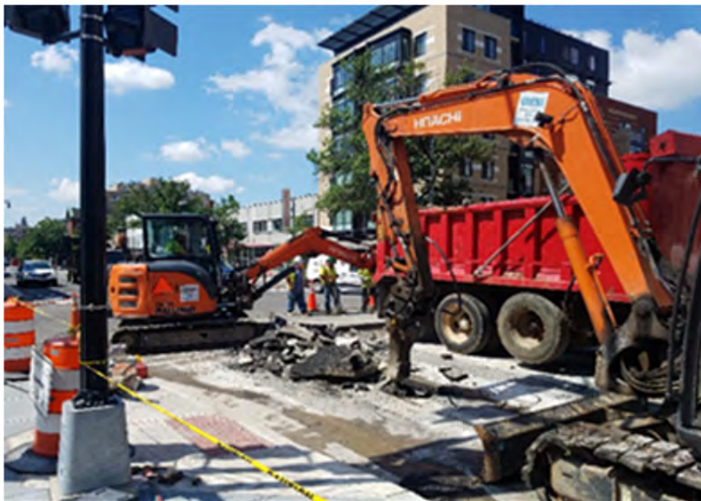
Demolition and excavation by Omni at NEC of 14 th & R St for 12" main work.
