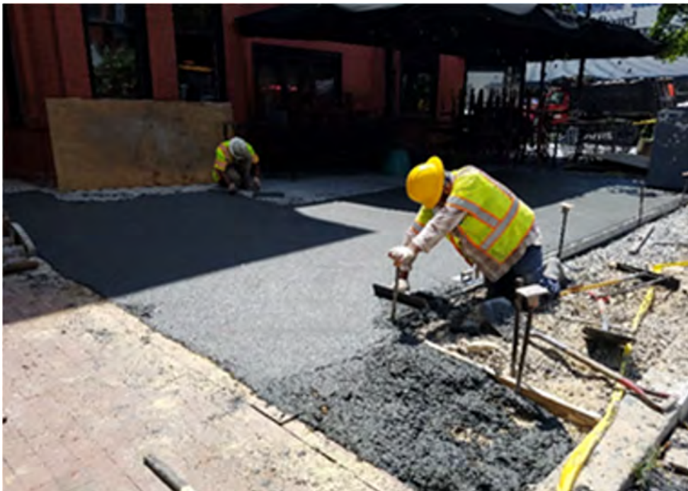
PCC sidewalk placement underway at NEC of 14 th & T St by D.E.N.
