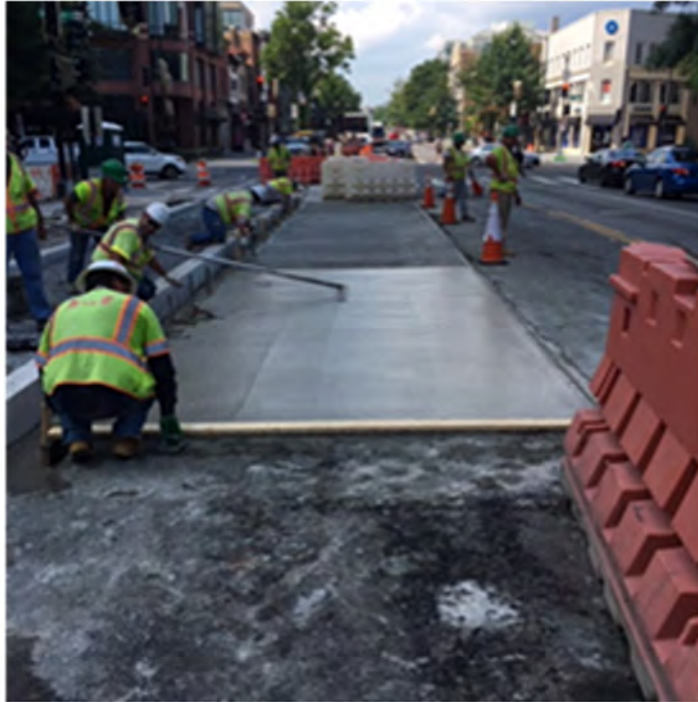
FMCC finishing up the concrete work for the installation of the Bus Pad at the southeast corner of 14th & Rhode island Street NW
