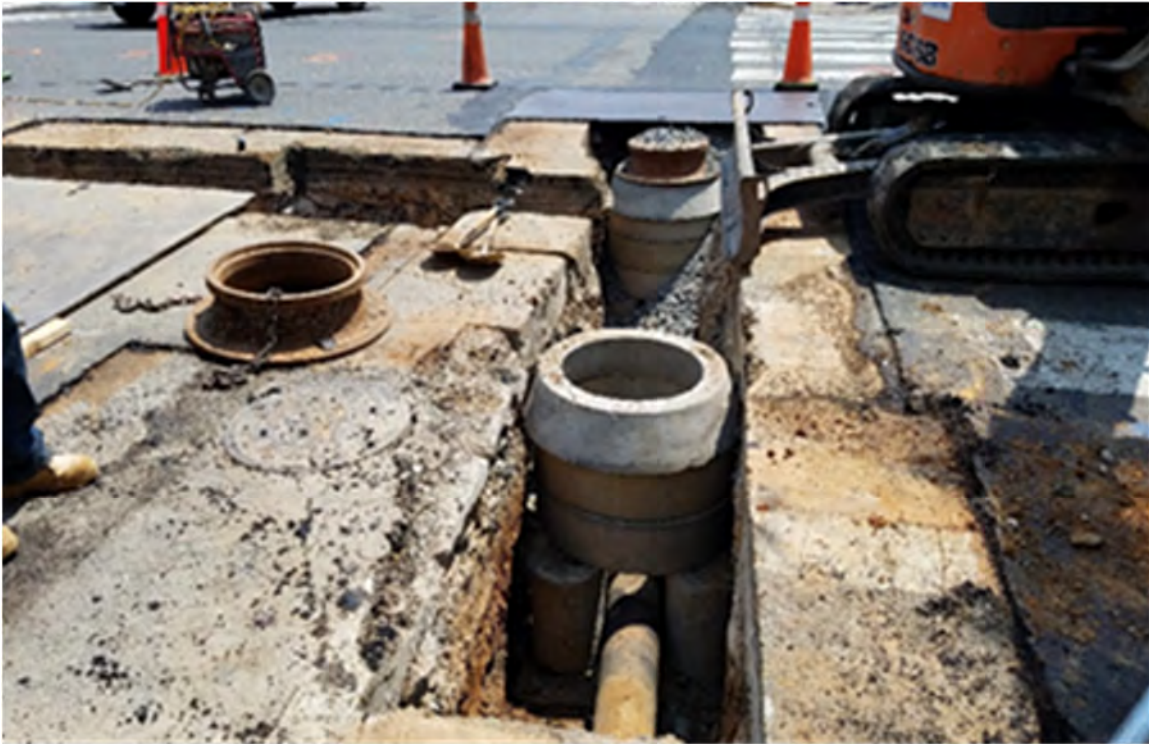
Valve casing for (2) 8" gate valves at R St trench.
